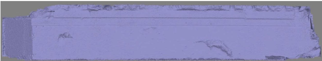
Figure 2-7: 3D Model of the Silverbell Bridge Box Beam Derived from Stereo Imagery.
