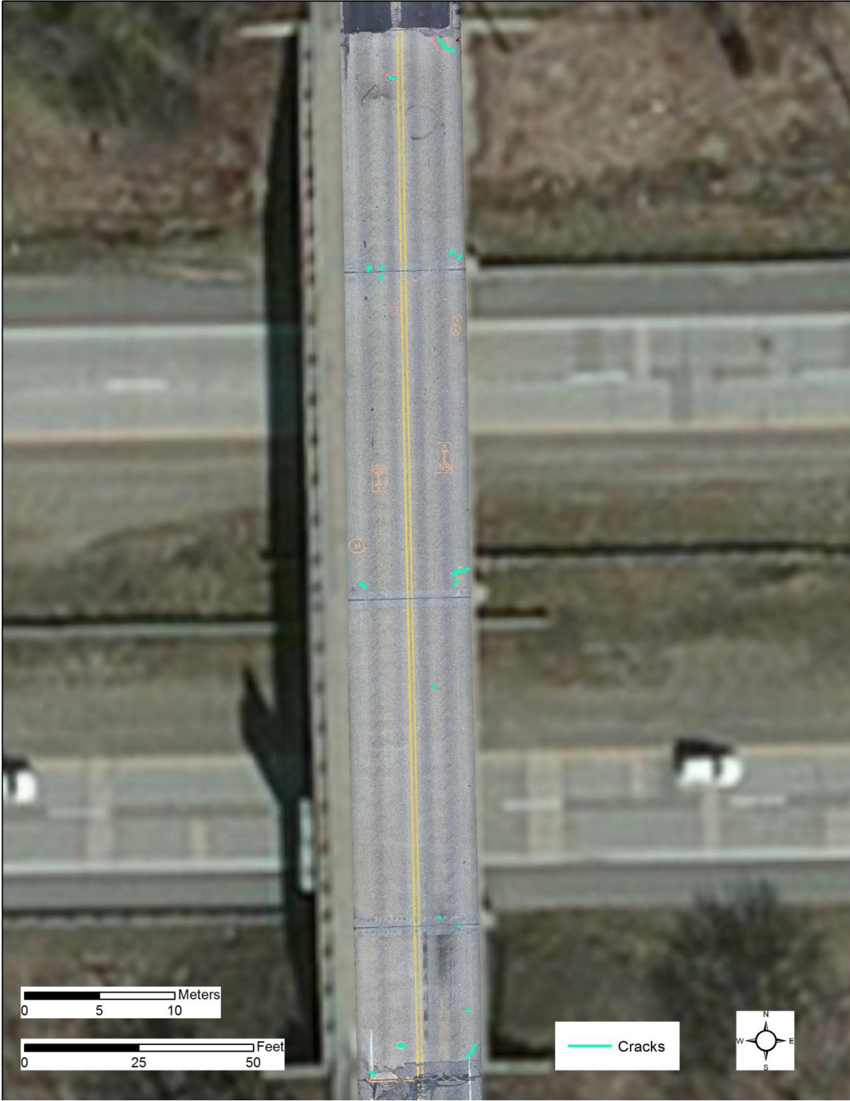
Figure 5-7: Detected Cracks on Maryland Ave.
