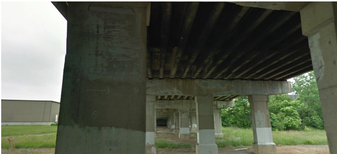
Figure 4-19: Current Condition of Bottom Deck Surface of Franklin Street Bridge.
