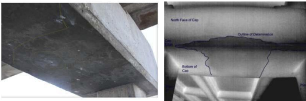
Figure 2-14: A) Visual Image of Marked Delamination on the Bridge Cap and B) Thermal IR Night Image of Delamination.
