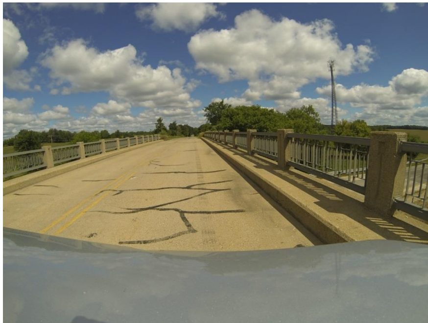
Figure 4-25: Example Image Captured on 24 Mile Road with a GoPro Mounted on the Hood of the Collection Vehicle.
