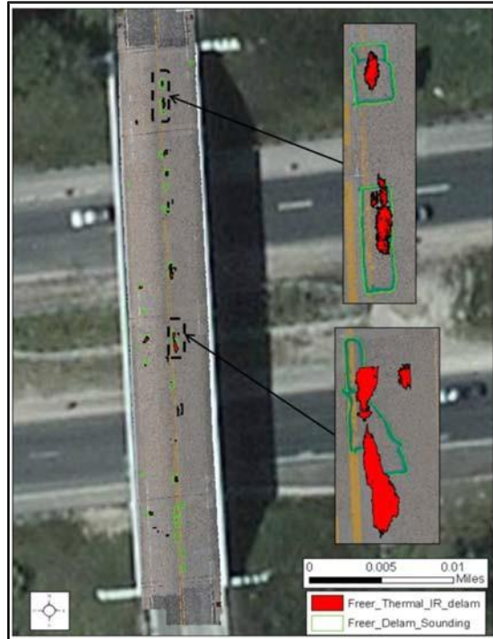
Figure 2-13: Combined Results of Thermal IR Imagery and Hammer Sound Inspection.
