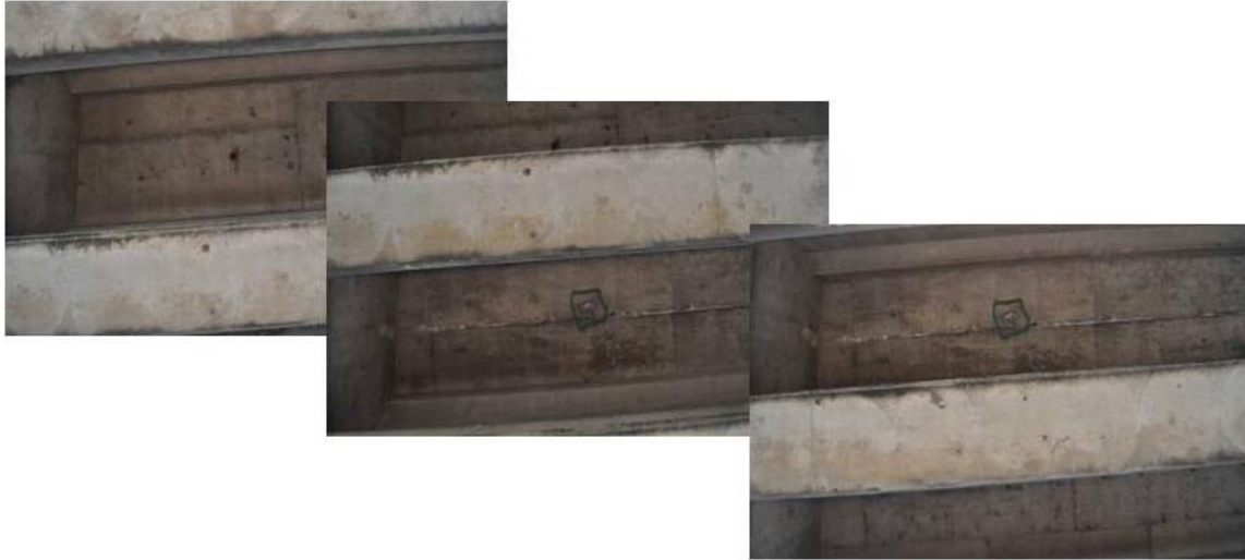
Figure 2-5: Photos taken with 3DOBS of the Underside of Willow Rd. Bridge (Ahlborn et al. 2012).
