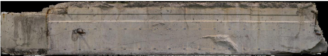
Figure 2-6: A Composite Image of the Silverbell Bridge Box Beam Derived from Stereo Imagery.
