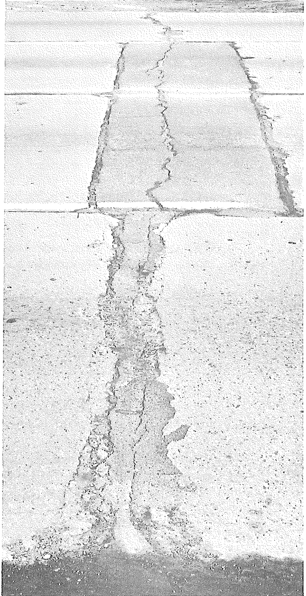
Joint Disintegration Station: 339+00 SB Roadway Age: 15 years
