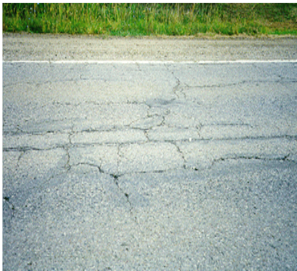
Figure 2. Typical pavement condition between Carsonville and Port Sanilac.
