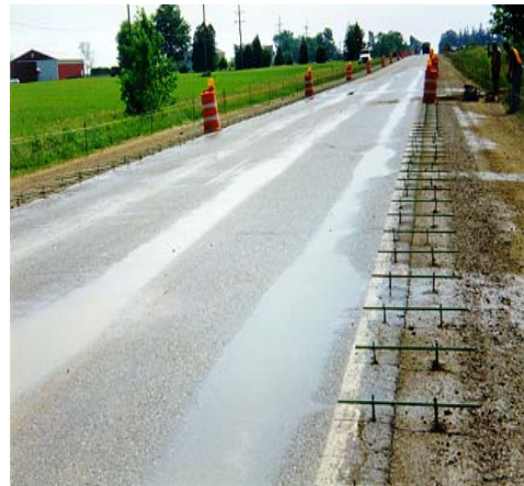
Figure 9. Water on bituminous just prior to paving. Note the rutting.
