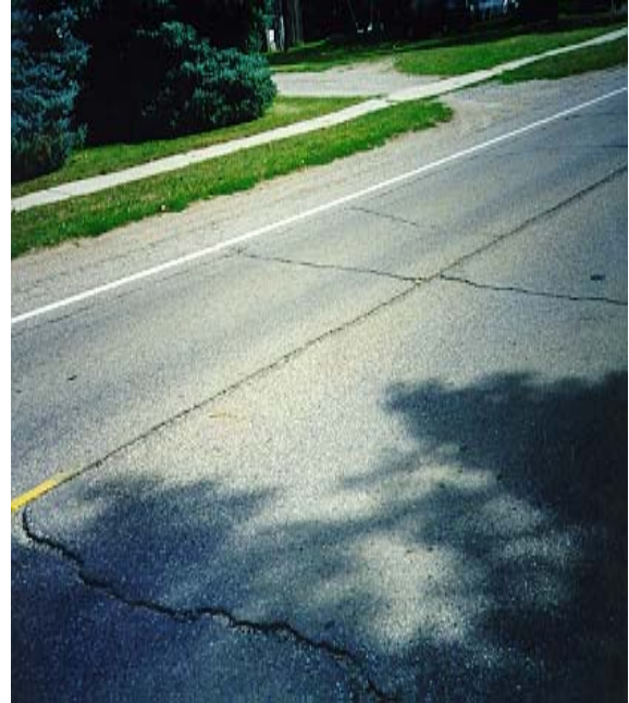
Figure 5. Typical pavement condition in Port Sanilac village limits.
