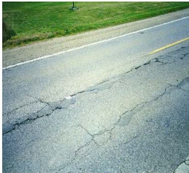
Figure 3. Typical pavement condition between Carsonville and Port Sanilac.
