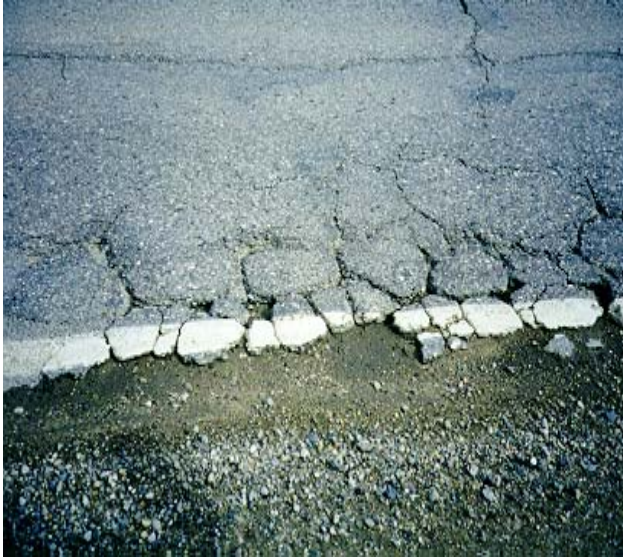
Figure 4. Typical edge deterioration.
