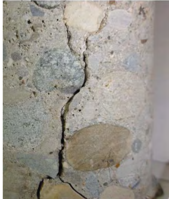
(b) Cracks on the core propagating from bottom surface to mid height
