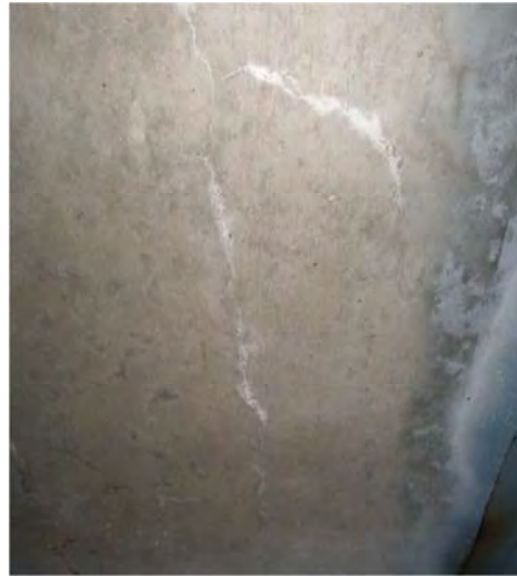
(b) White traces and cracks (tail span)
