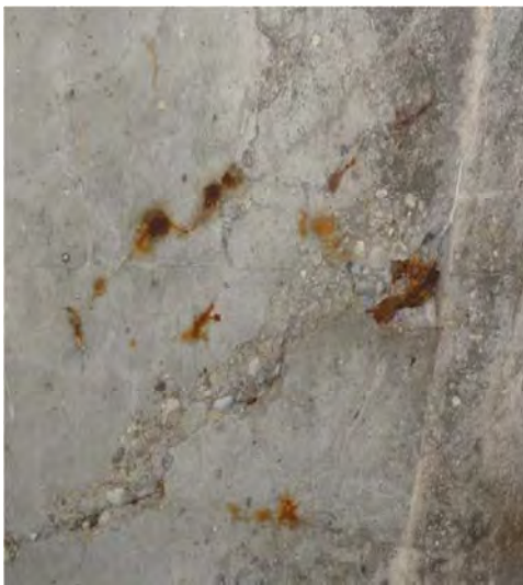
(c) Cracks and corrosion traces (tail span, WB)
