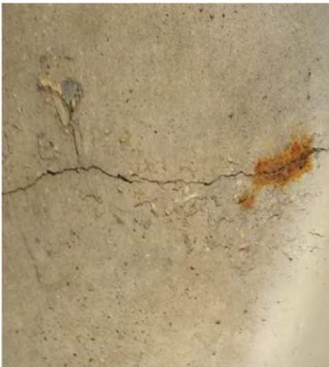
(c) Transverse bottom cracks (Scale \approx 1:20 ) (tail span)
