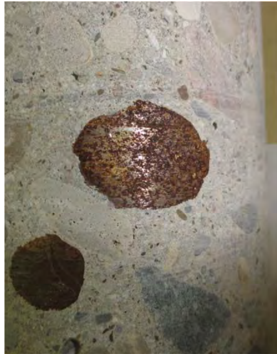
(b) Rust on the reinforcing steel
