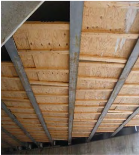
(a) Plywood cover on most part of the bottom deck of 63022-S01 carrying I-96 over Kent Lake Road
