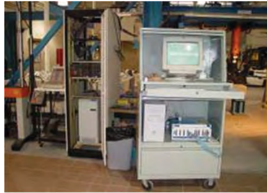
(b) Controllers and data acquisition
