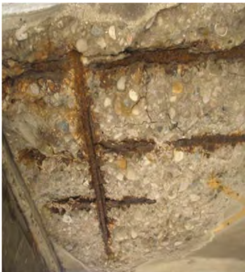
(c) Deteriorated concrete and exposed reinforcement (under plywood)
