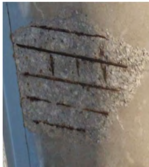
(d) Deteriorated concrete and exposed reinforcement bar (tail span, WB)
