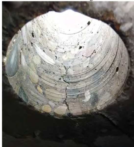
(d) Crack on deck propagating from bottom surface to mid depth
