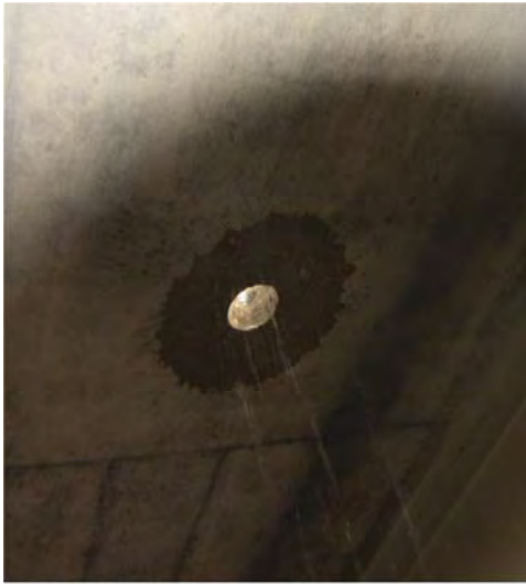
(c) Resulting hole in concrete deck
