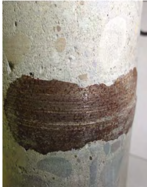
(b) Rust on the reinforcing steel
