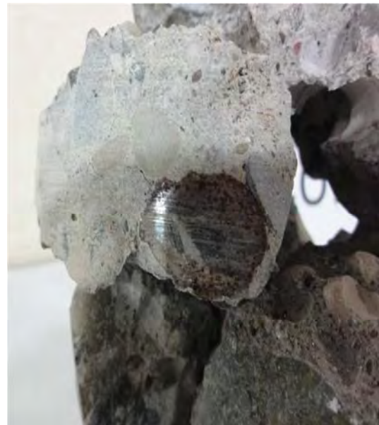
(b) Rust on the reinforcing bar
