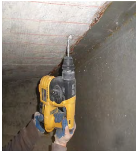
Figure 4-3 Exposing reinforcement bar
