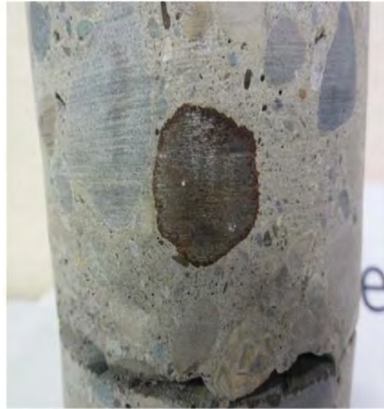
(b) Rust on the reinforcing steel
