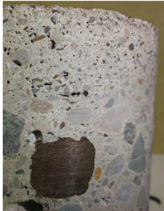
(b) Rust on the reinforcing steel
