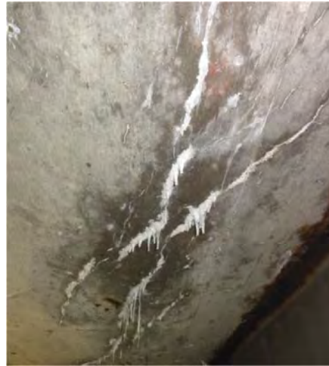
(b) Crack and efflorescence (tail span, WB)
