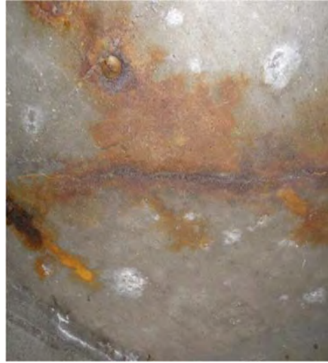
(b) Rust traces and cracks (tail span)
