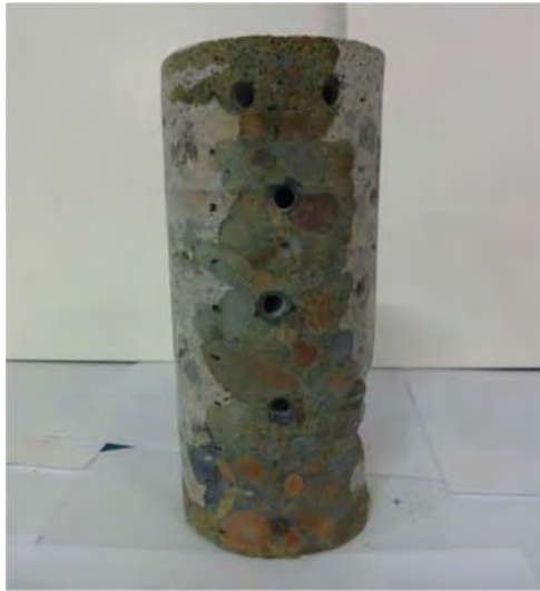
Figure 6-9 63022-S01 carrying I-96 WB over Kent Lake Road core exposed to Rainbow Indicator
