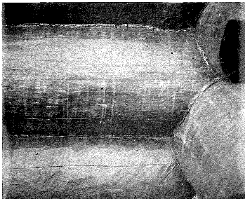
Figure 9. View of inside wall showing insect borings, sole evidence of any deterioration within the lodge.
