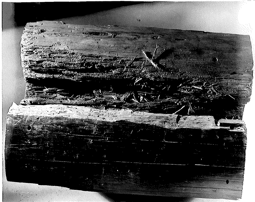
Figure 10. Portion of section removed for study showing insect borings in exterior wall surface.
