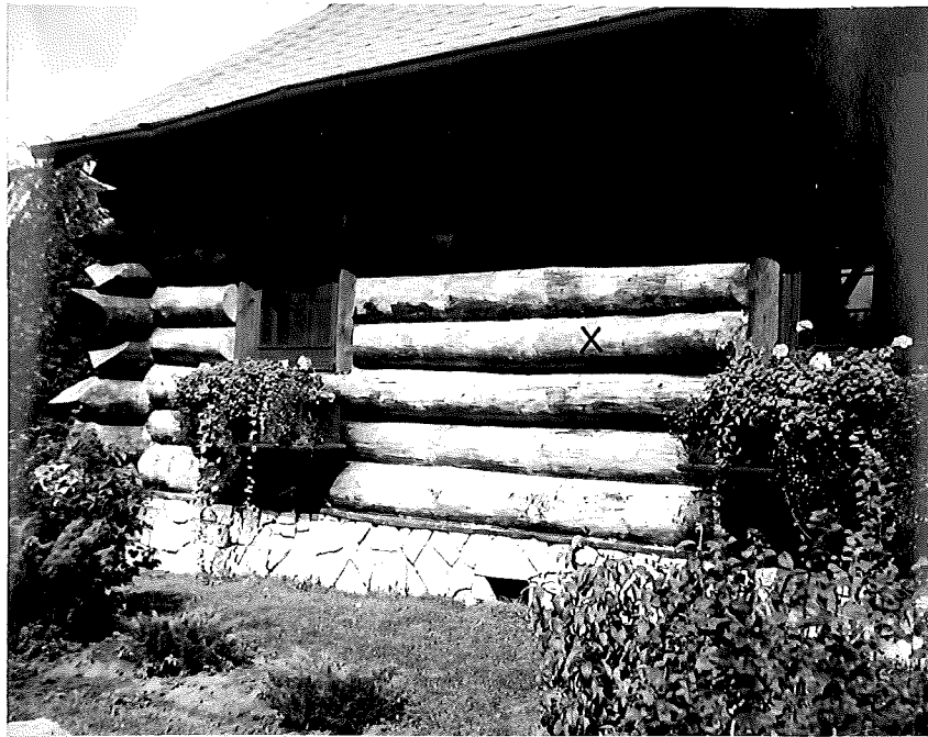
Figure 3. Portion of south wall. Sample removed at point marked "X".
