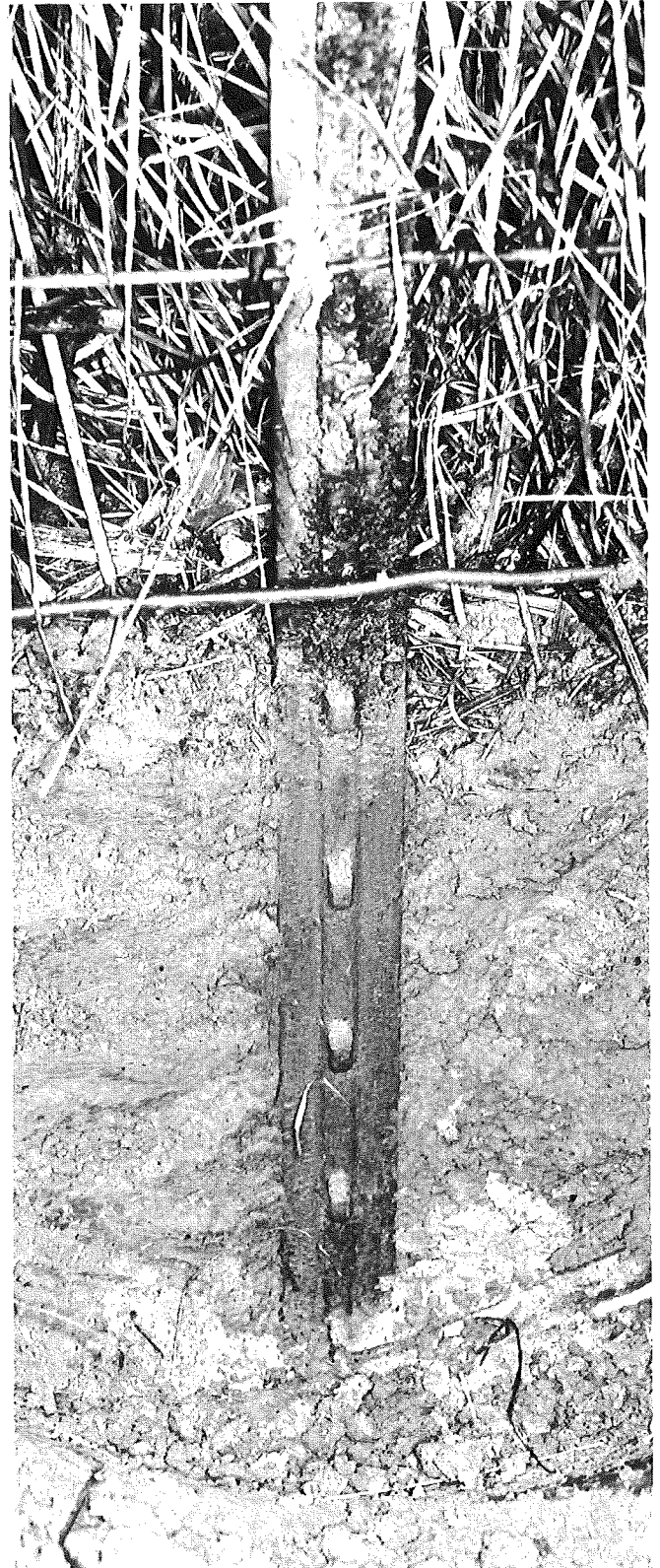
Figure 17. Age: 5 years. West side of I 75 at Vreeland Road overpass. Clay loam soil. Green paint excellent below ground level with practically no apparent corrosion. Severe corrosion at ground line, less severe above ground.
