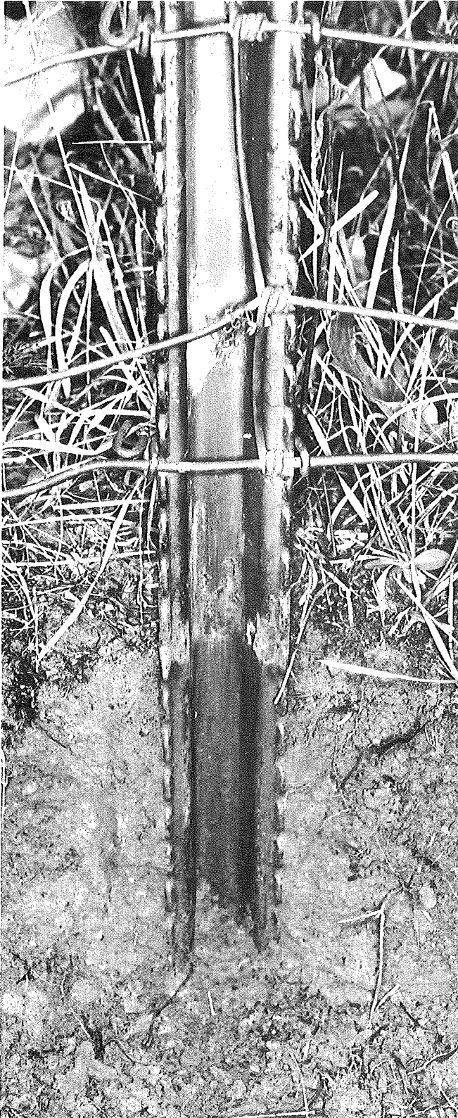
Figure 18. Age: 5 years. West side of I 75 at Mount Morris exit. Sandy loam soil. Green paint excellent below ground level with little apparent corrosion. Severe corrosion at ground line, less severe above ground. White area is caterpillar's nest.
