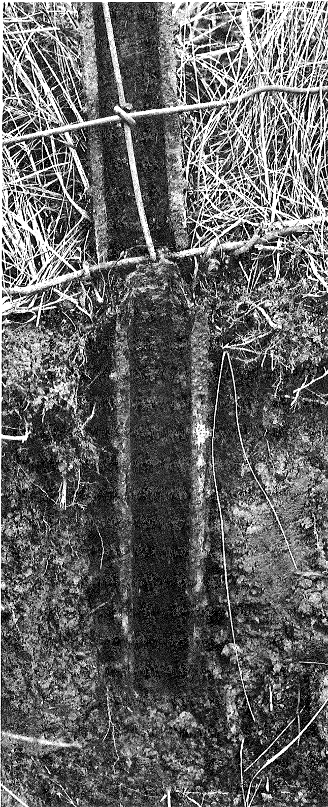
Figure 24. Age: 39 years. North side of US 16 just east of Fowlerville. Clay and loam soil, stony. Corroded entirely through at ground level. Apparently protective rust has formed below grade. Corrosion severe above ground.
