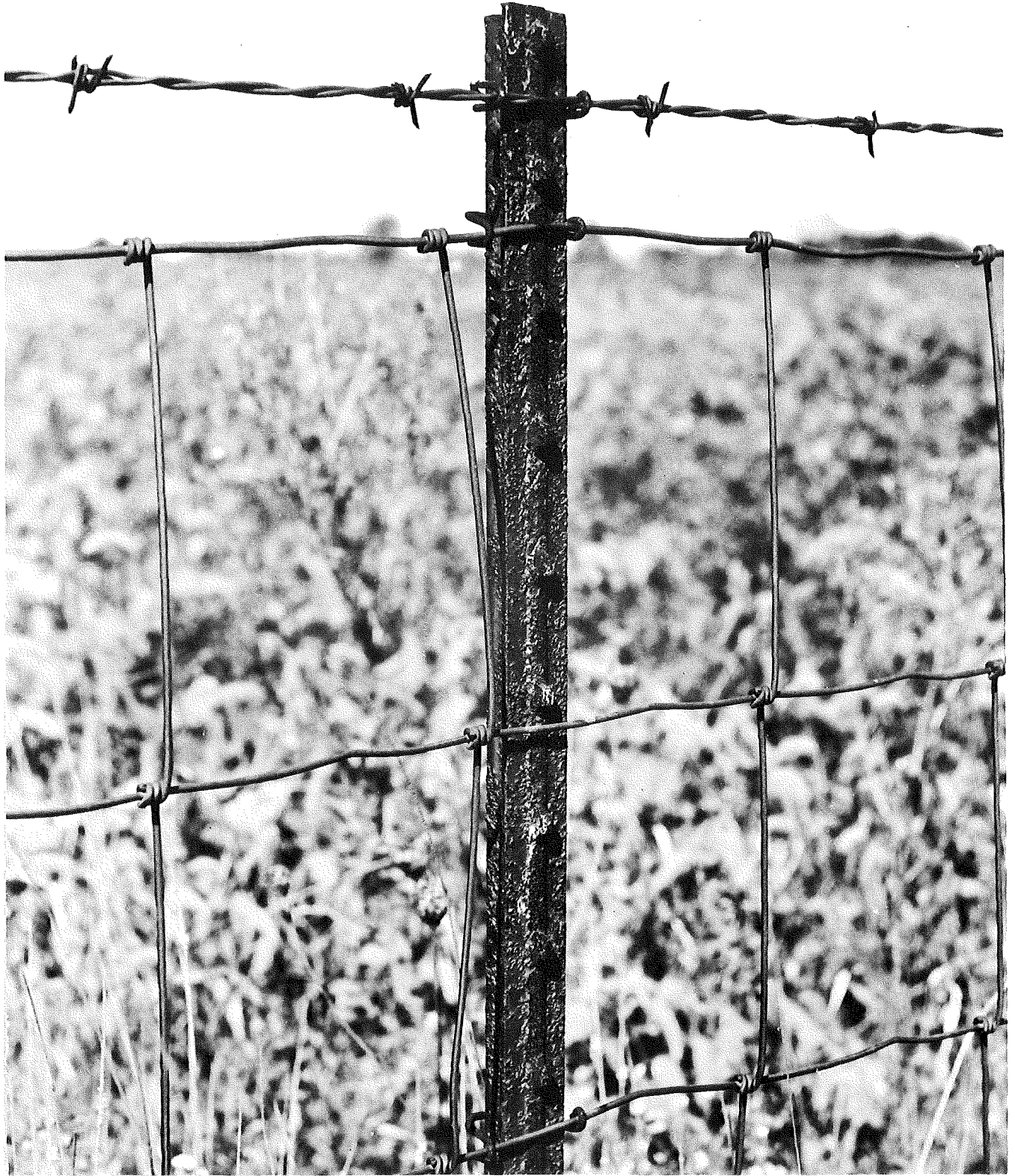
Figure 7. Age: 5 years. West side of I 75 at Vreeland Road between Detroit and Monroe. Excessive, severe corrosion, typical of posts in this area. Post is still structurally sound, but wobbly.
