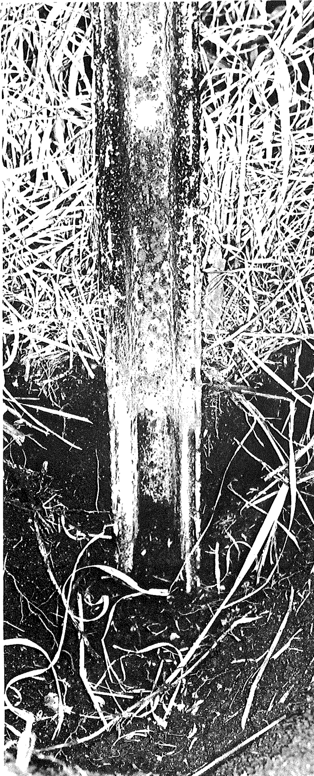
Figure 20. Age: 8 years. North side of I 94 just west of US 127. Black dirt. Yellow paint still in good condition below ground level, with little corrosion. Intense corrosion at ground line with severe corrosion above ground.
