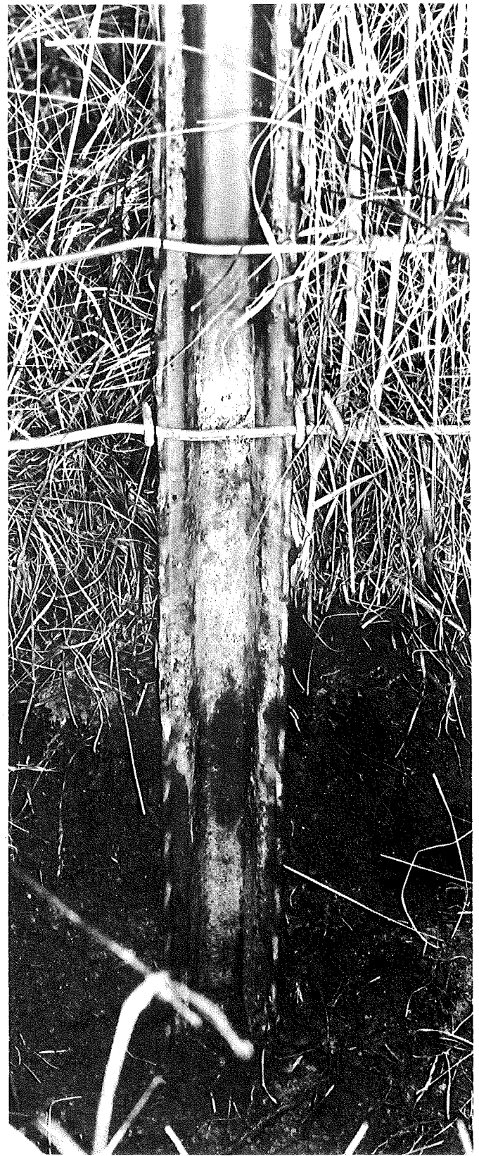
Figure 15. Age: 4 years. East side of I 75 south of M 57. Dark, rich soil. Green paint still satisfactory below ground but corrosion is severe at ground level.
