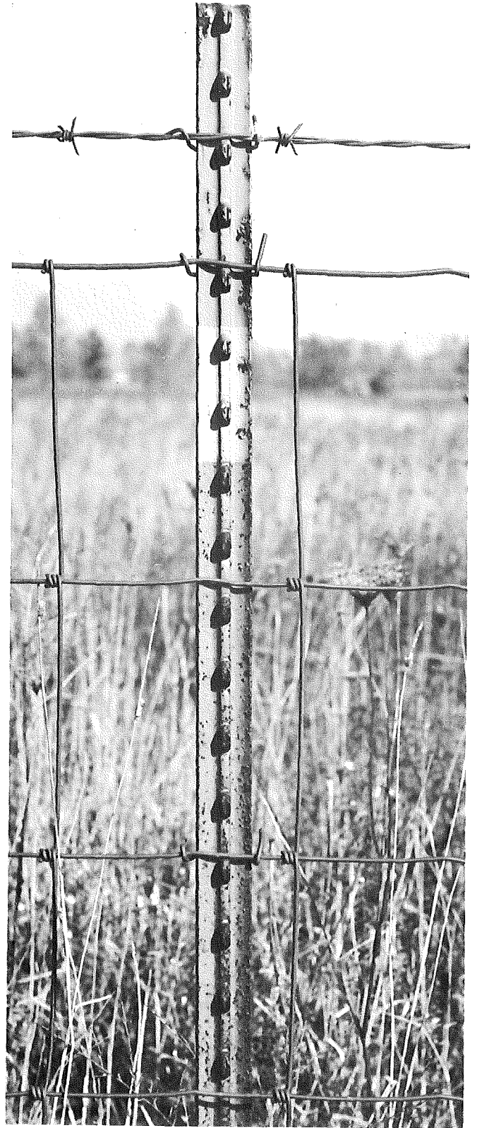
Figure 4. Age: 3 years. North side of I 94 just west of Kalamazoo, east of Oshtemo exit. Red paint. Localized beginning corrosion.
