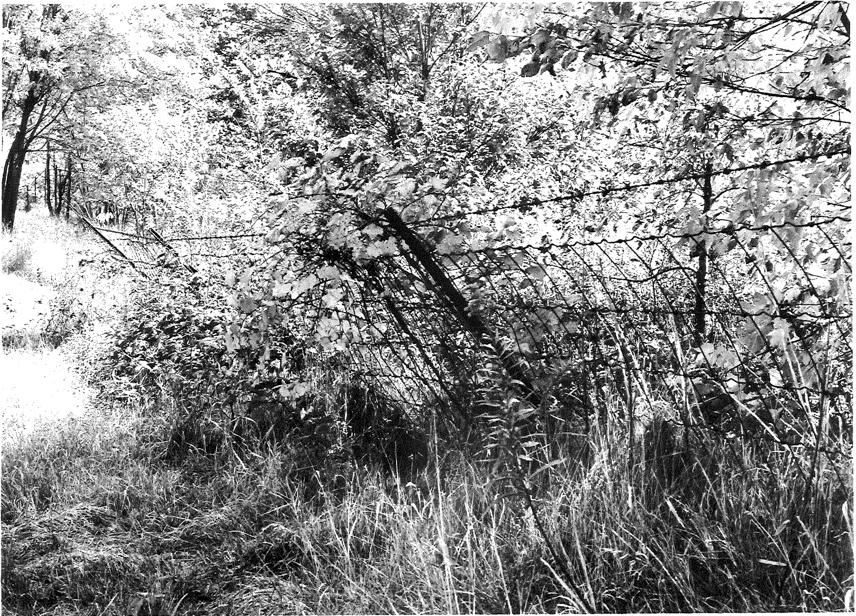
Figure 8. Age: 13 years. South side of I 94, 1/2 mile east of Cooper Street exit, Jackson area. Large section corroded through at ground level, with fence lying on ground. One post (see Figure 9) taken to laboratory for study. Wire fencing badly corroded.
