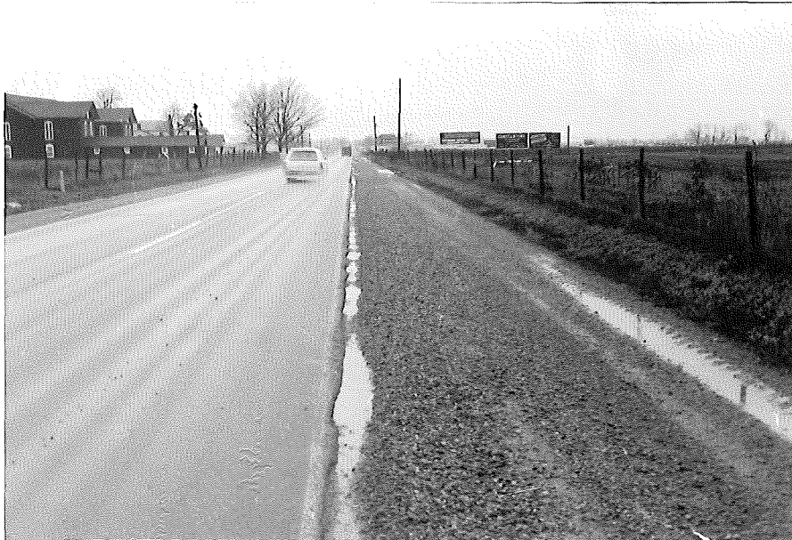
Deep rutting and edge of roadway break up (US-131 S. of Constantine - 20-ft roadway)
