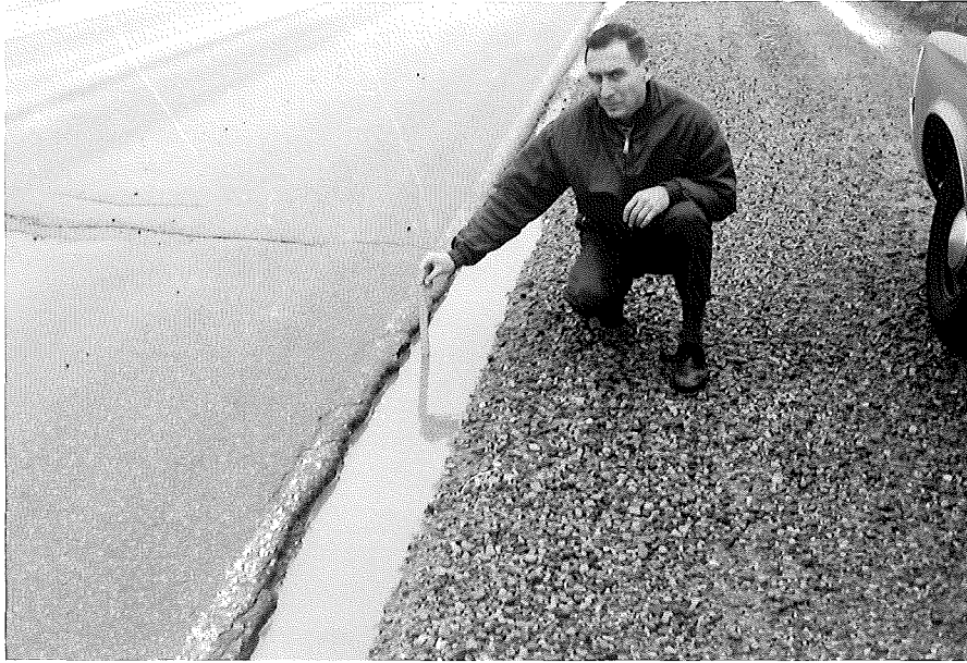
Deep rutting and edge of roadway break up due to undermining (US-131 S. of Constantine - 20-ft roadway)
