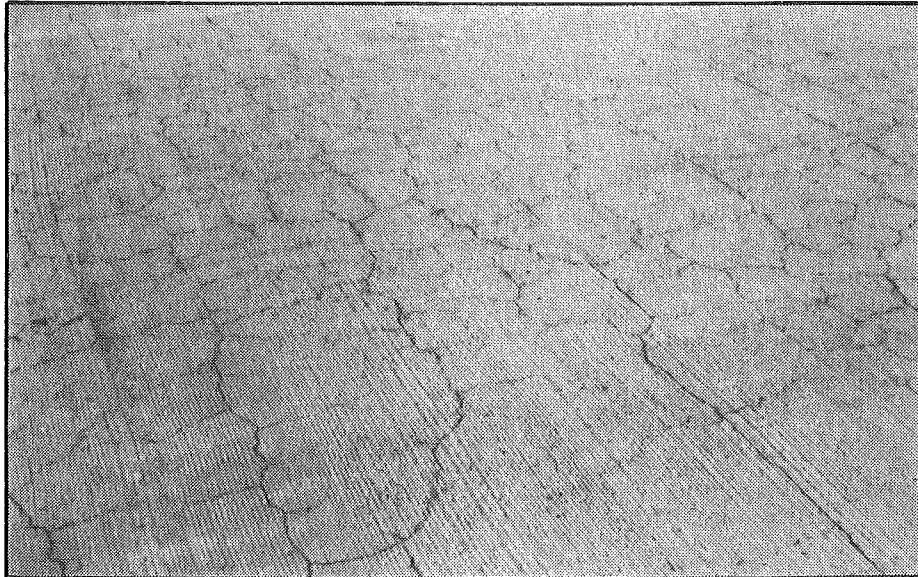
Figure 7. Random crack pattern in eastbound I 96 inside lane of LSHD pour of 1975 on S10 of 47065 after seven years.
