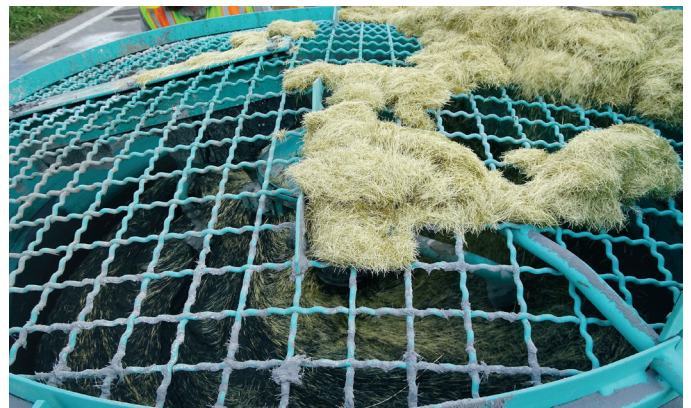
Near the end of the MI-UHPC mixing process, crews add steel fibers through a grate over the mixing barrel.
