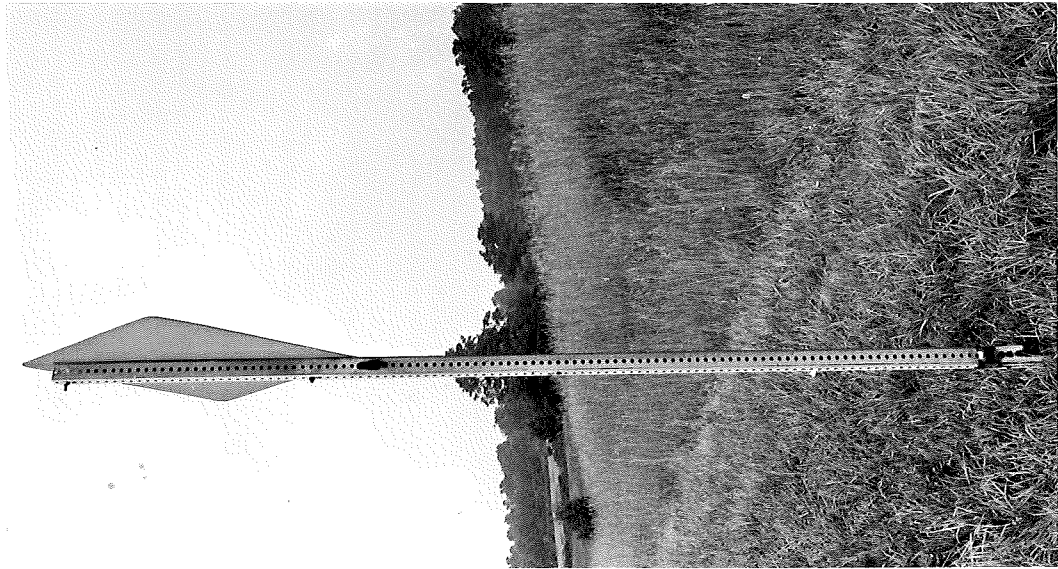
Figure 2. Six-year old post on west-bound I 96 west of Grand River Ave shows insignificant loss of coating except at contact points (sign and boot) and is representative of the majority of these installations.
