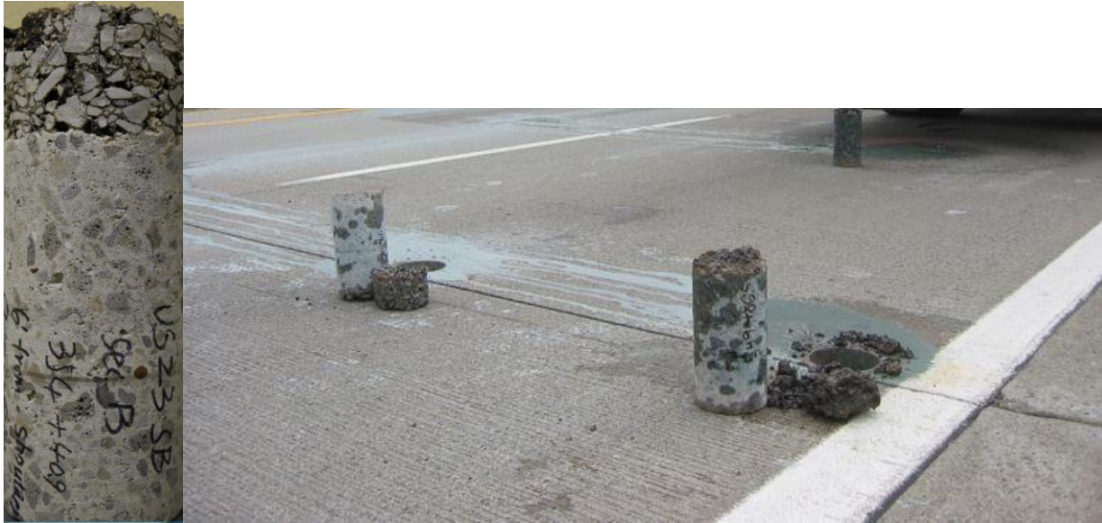
Figure 2.11. (a) Close-up of bonded ATPB away from joints and (b) and partly eroded ATPB at outer corners
