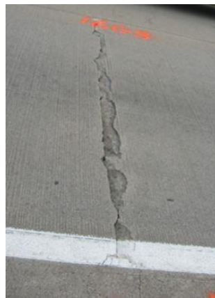
Figure 2.13. Typical crack spalling in section B (2006)
