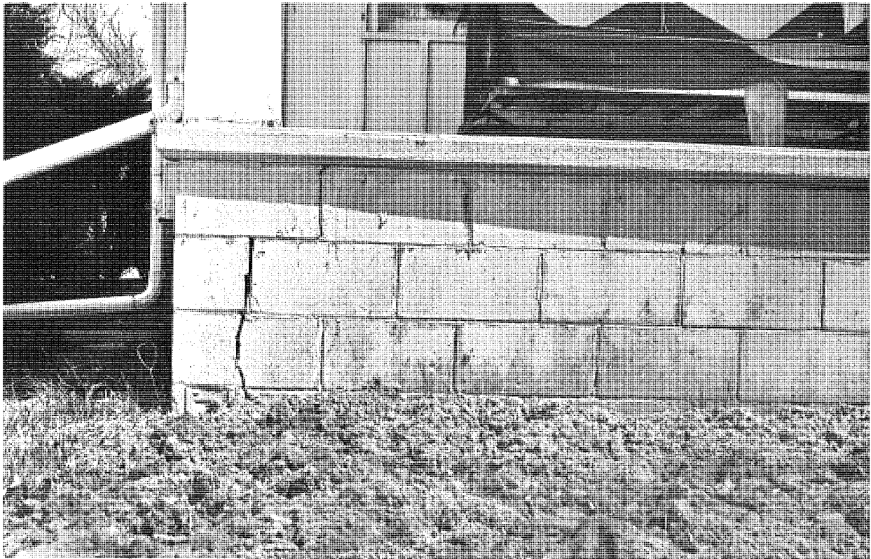
Figure 1. Condition of porch foundation showing cracking at the southeast (upper) and southwest (lower) corners.
