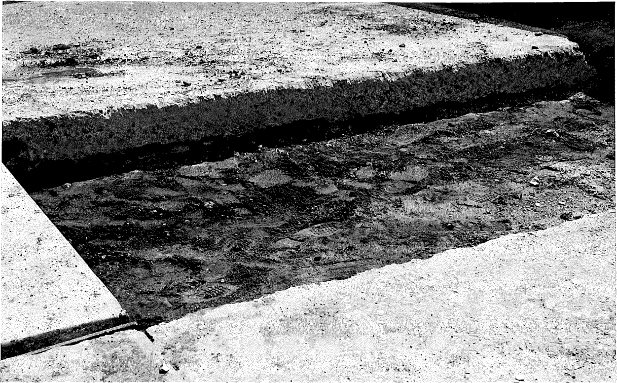
Figure 3. Typical condition of Vermeer sawcut.
