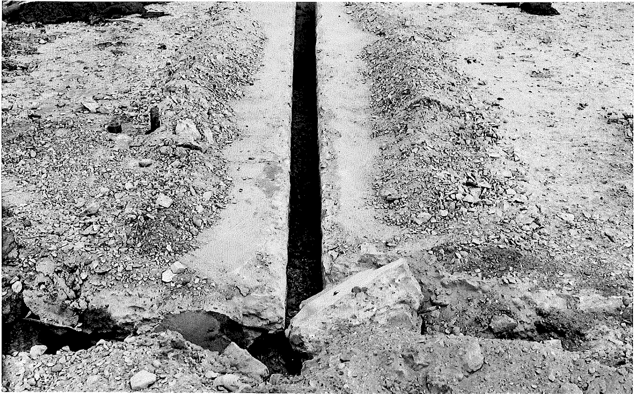
Figure 1. Vermeer sawcut on south side of repair in passing lane. Corner spall can be seen to the right of cut.
