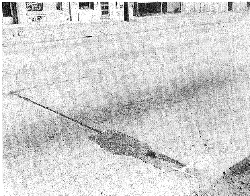
▲ FIGURE 2 B. LOCATION OF GRID BREAK 6. IN CONCRETE PAVEMENT.
