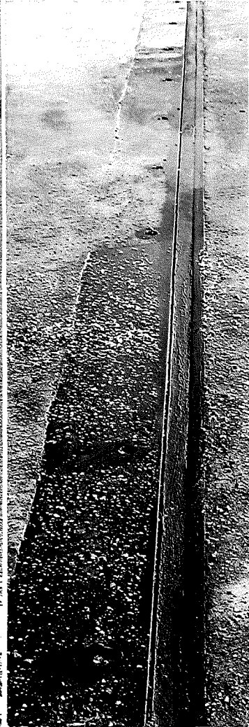
Figure 3. Polysulfide sealer shows adhesion loss on leading edge of bridge expansion dam after three months of winter service.
