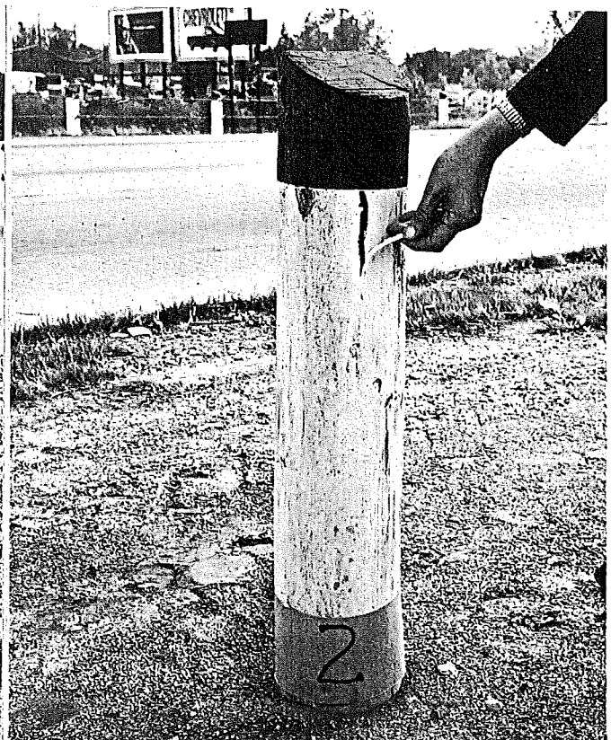
Figure 3. Breathing white paint exhibited staining and could be peeled off untreated post after almost two years of service.
