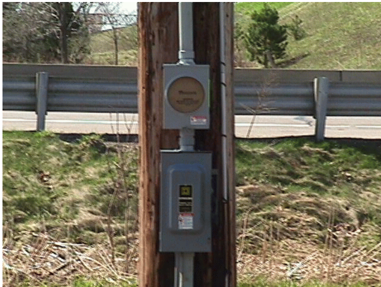
Figure 5 Meter Socket not installed until 4/15/99.
