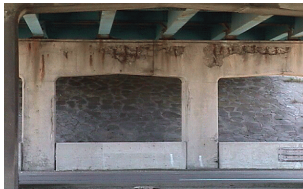
Figure 1 Effects of corrosion upon the substructure (Jackson, Michigan).
