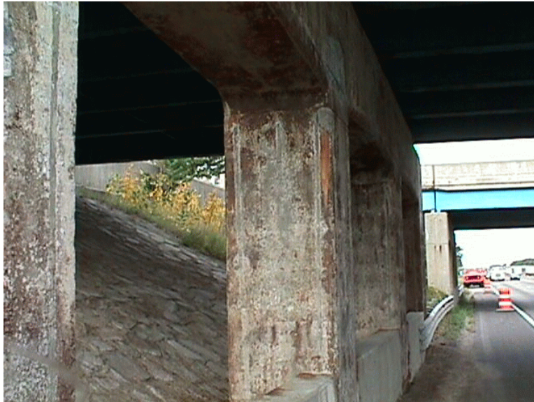
Figure 9 Rust Stains from the ECE Process
