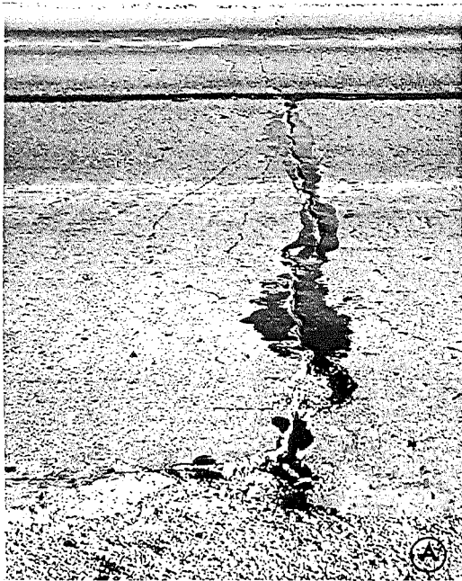
▲ STATION 653 +65. SEALED WITH BRAND A. NOTE LOSS OF SEALING MATERIAL.
