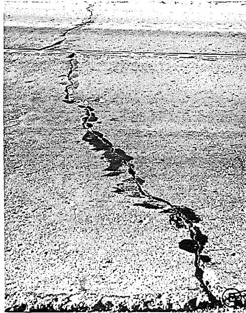
▲ STATION 651 +85. ANOTHER OPEN CRACK SEALED WITH BRAND A AND SHOWING LOSS OF MATERIAL.
