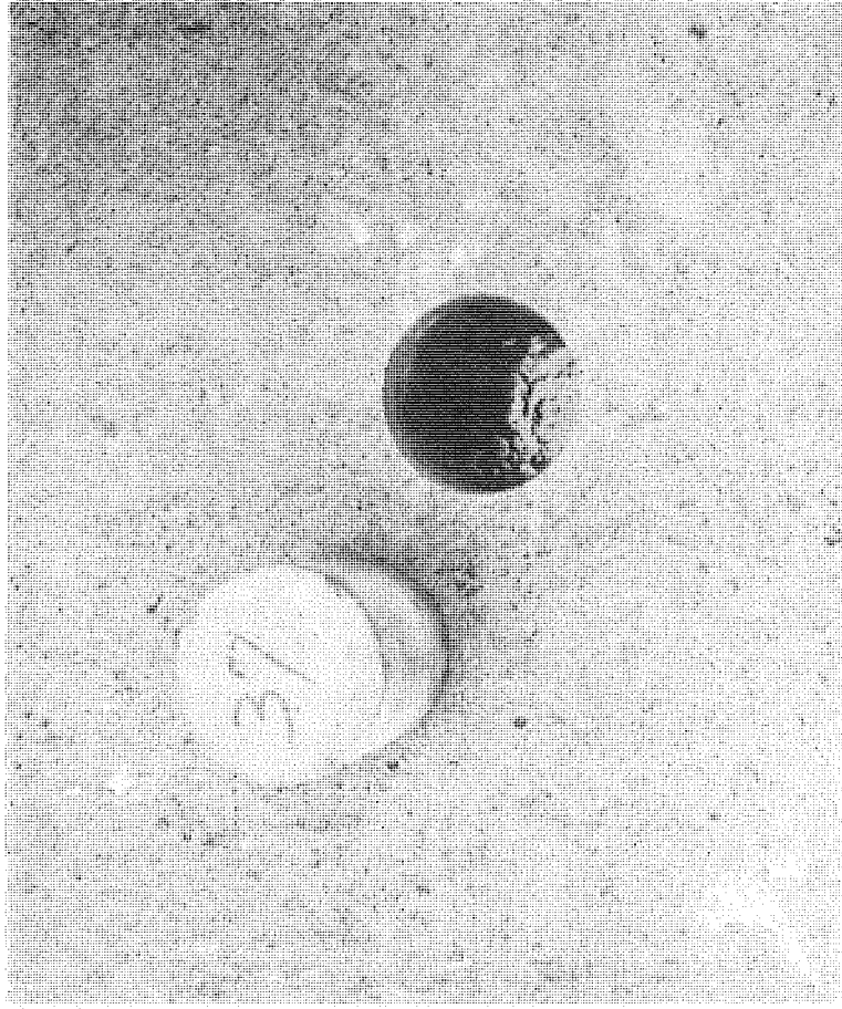
Figure 4. Free water, seen at the bottom of the core hole, is located about 9 in. from the pavement surface a day after a summer shower.
