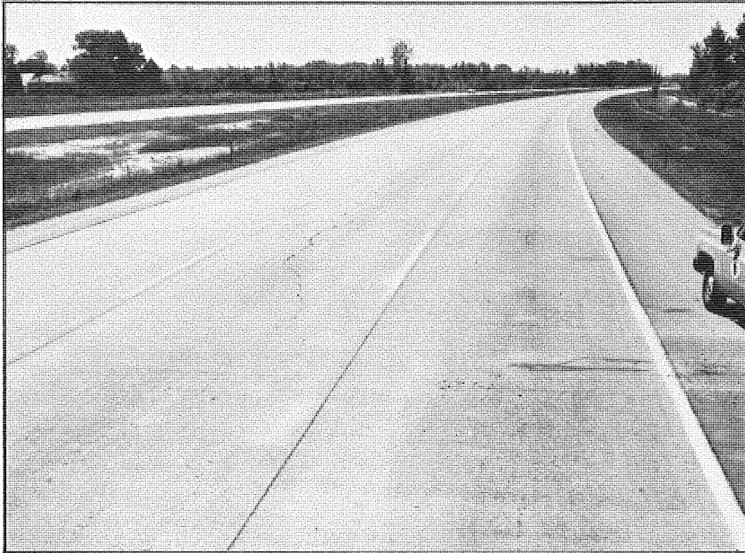
Figure 14. Longitudinal cracking not related to 'frost tenting' action.
