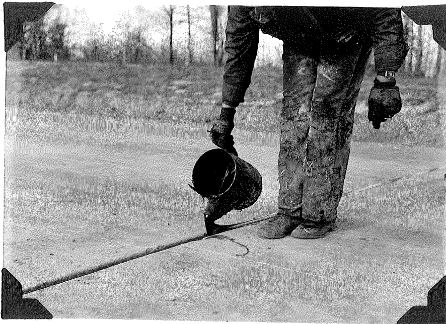
B. Pouring Asphalt-Latex Joint-Sealing Compound (Note rubbery consistency of the material.) Design Project - Michigan Test Road. Photograph taken October, 1940
