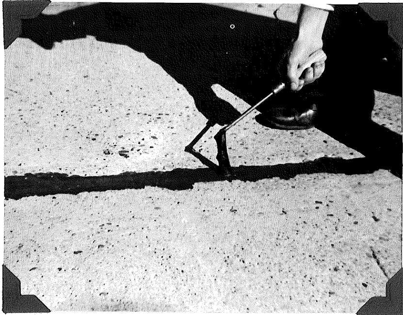
C. General Plasticity of the Joint Seal Material Illustrated in "A" after 3 Years in Service. Temperature 50°F. Photograph taken October, 19, 1944.
