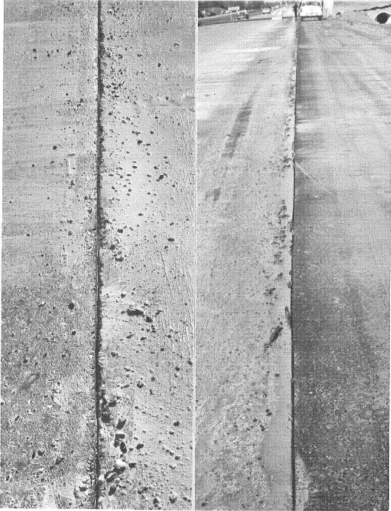
Figure 13. After sawing (left), the longitudinal joint is flushed with water, then cleaned and dried with compressed air.
