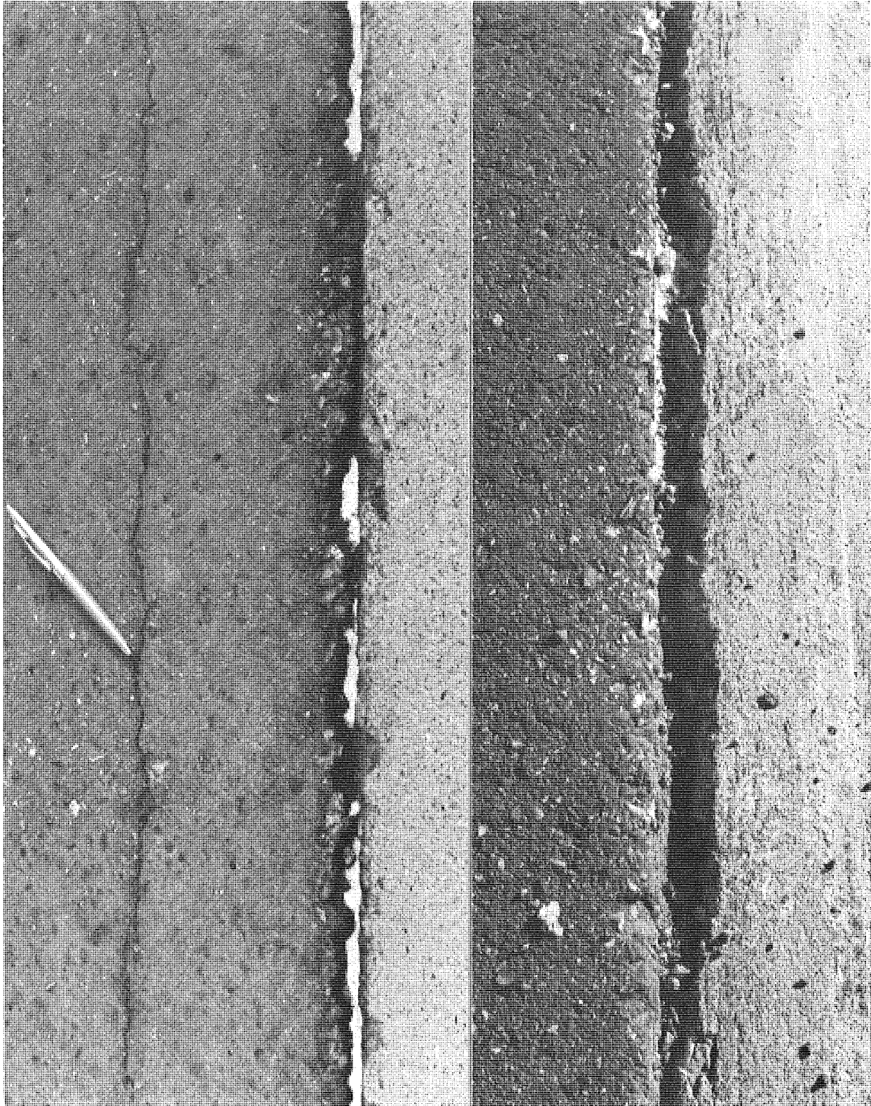
Figure 3. Typical splitting away of conventionally constructed bituminous shoulders from concrete pavement at two Project 2 locations, leaving opened joints wide enough for infiltration of water, sand, gravel, salt, or other incompressible material resisting normal joint movement. At left, typical longitudinal crack has developed parallel to open joint. Photographed 4 months after construction (May 1963).
