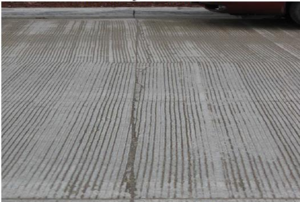
Transverse Crack 100' north of Pearl NB-1
