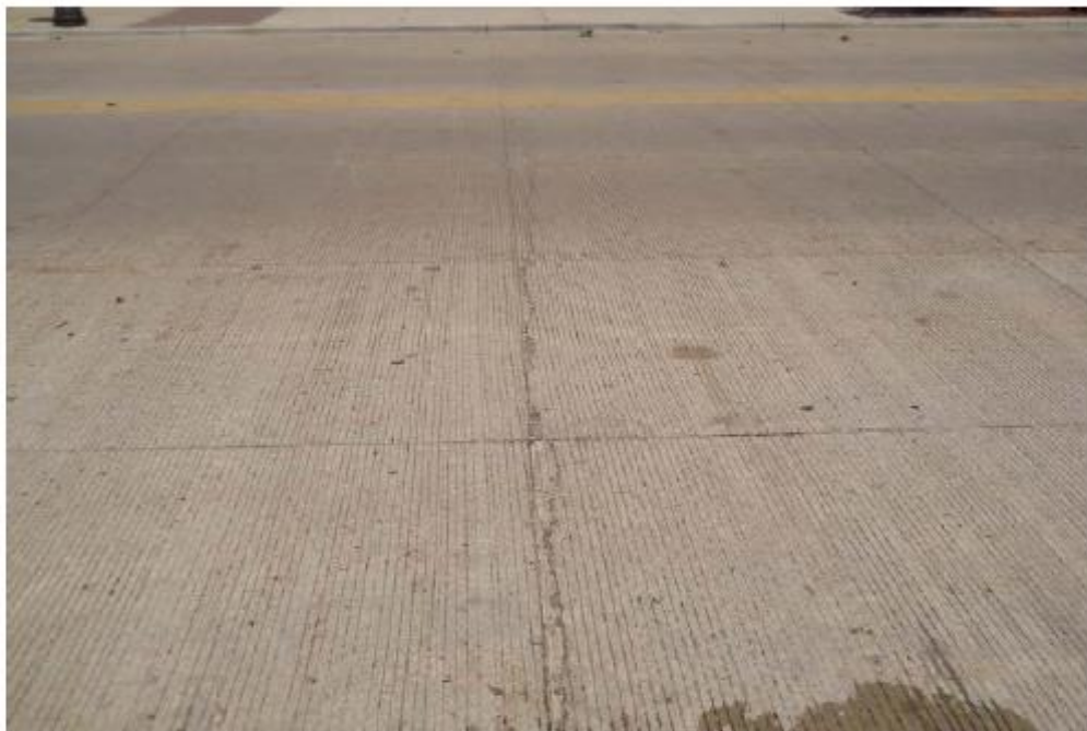
Picture #8: Transverse crack near joint.
