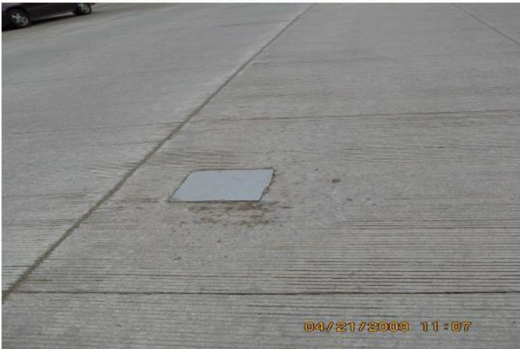
Scaling around patch in CL near 136 Main Street
