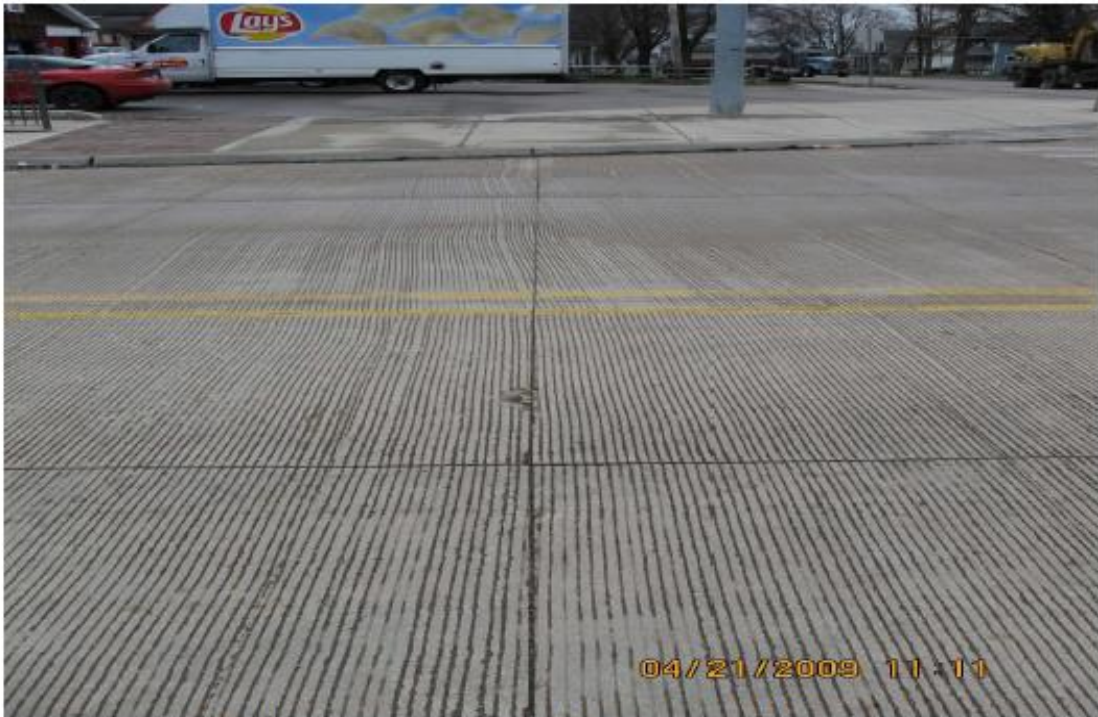
Spall near springpoint of Maple/M-99 NE quad
