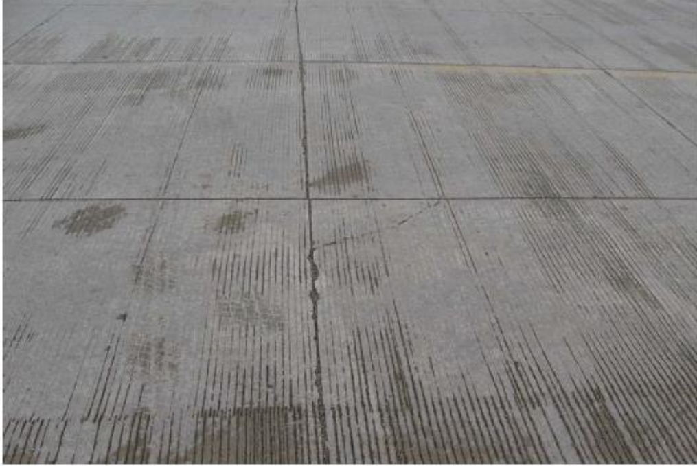
Corner Cracking 64' from POE NB-1
