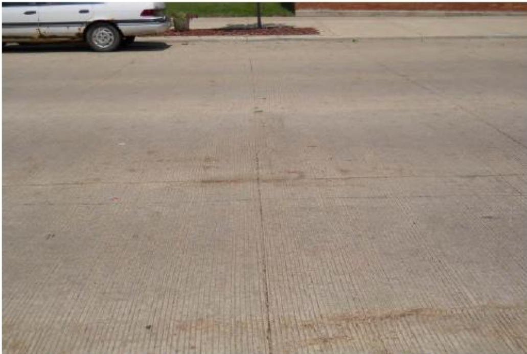
Picture #12: Transverse crack, parallel with joint.
