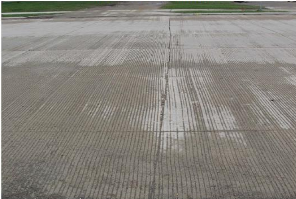
Additional cracking near POE NB-1
