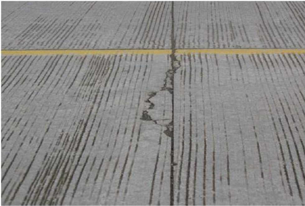
Spall 30' north of Pearl St. SB-1
