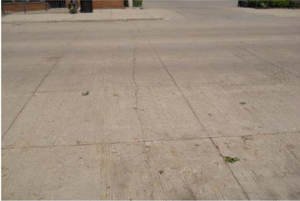
Picture #13: Mid-panel transverse crack.
