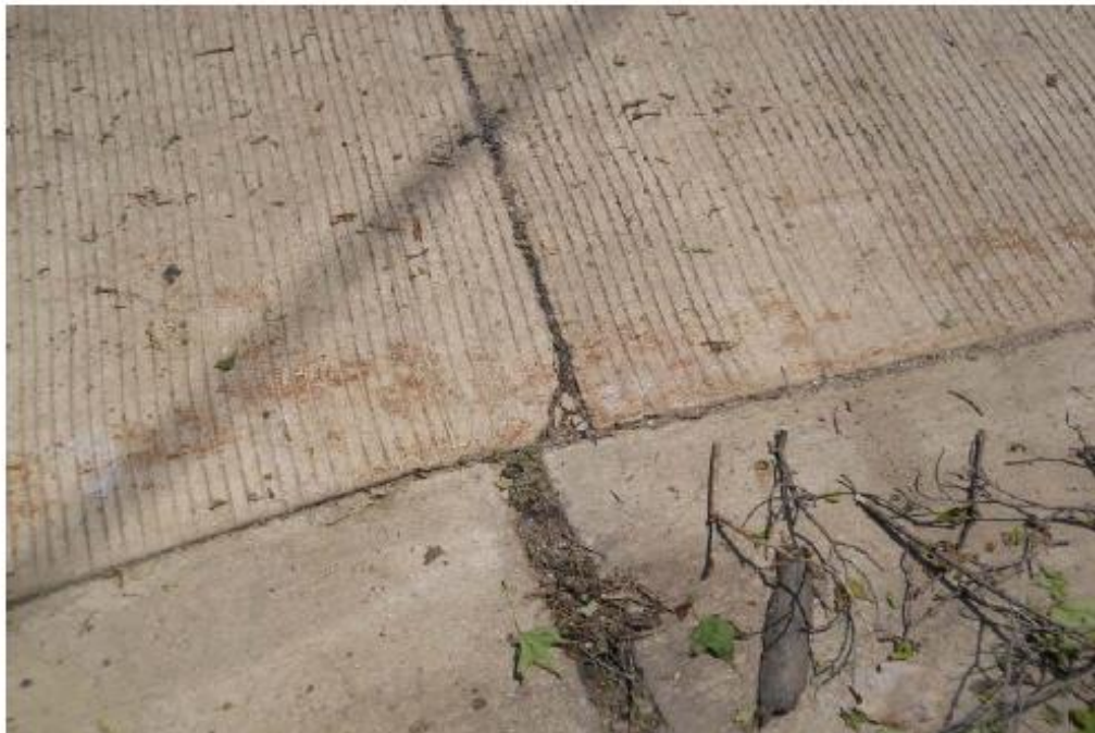
Picture #2: Corner spall near gutter pan.
