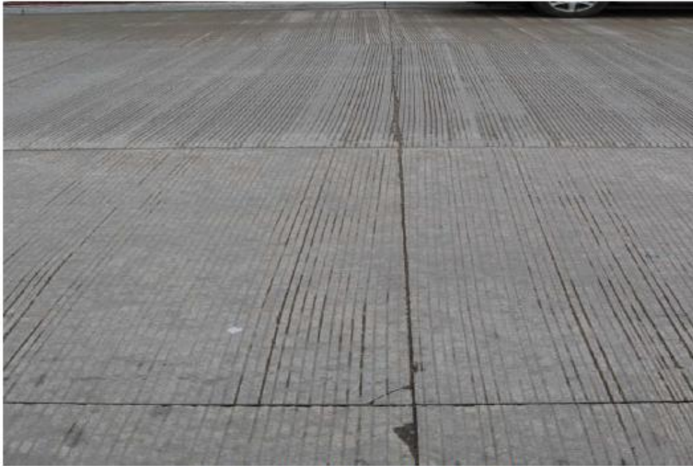
Corner Cracking 100' north of Pearl SB-1
