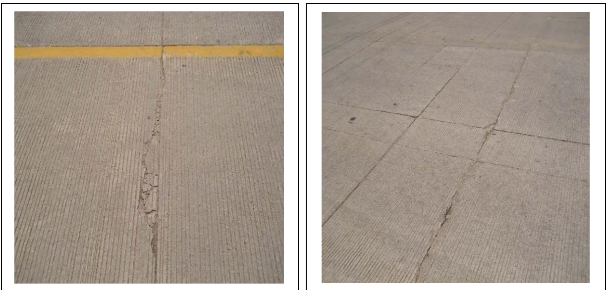
Figure 9. Joint Spalling and Transverse Cracks on M-99 from MDOT Warranty Report SWAD 2870 (2011)
