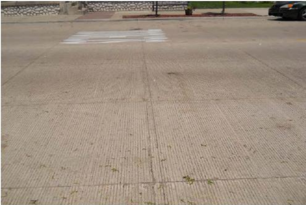
Picture #10: Transverse crack near joint.
