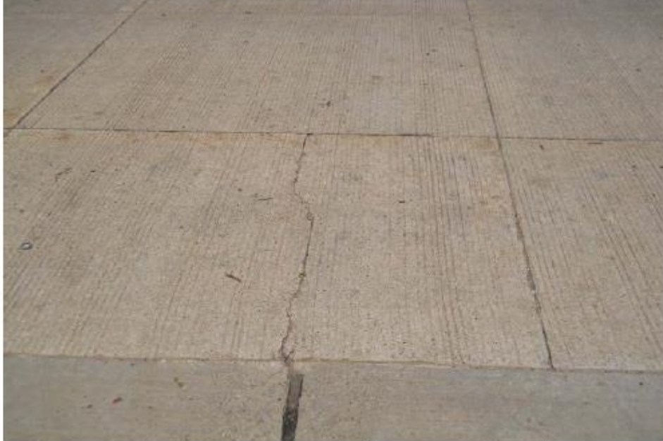
Picture #21: Transverse crack near curb and gutter.
