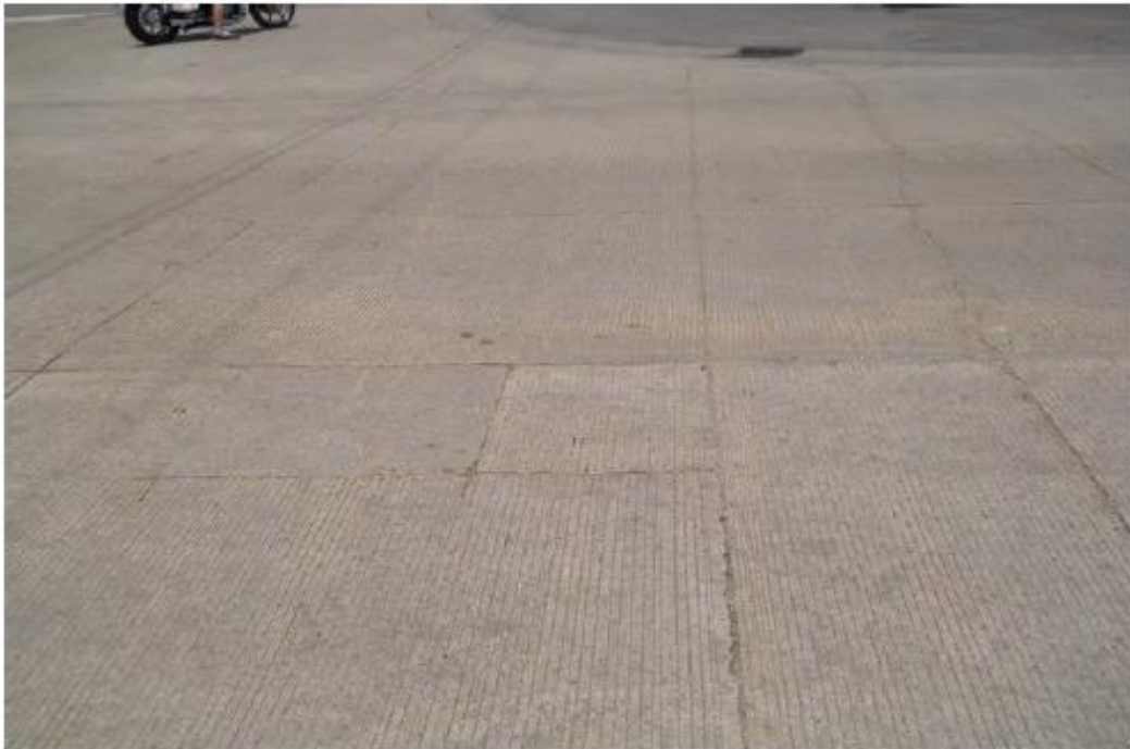
Picture #18: Longitudinal crack extending from previous patch.
