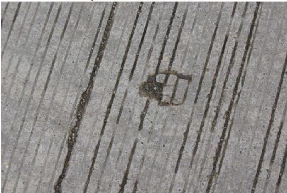
Spall 80' north of Pearl St. SB-1
