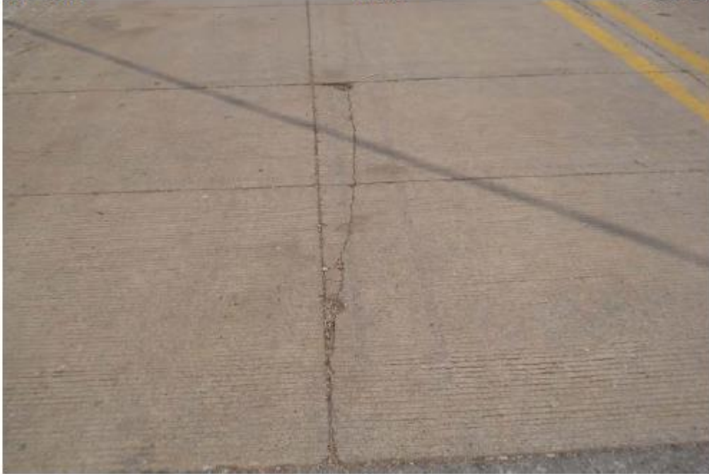
Picture #3: Longitudinal cracking (two panels).
