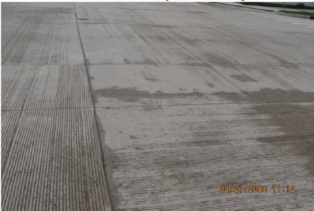
Transverse Crack North leg of M-99/Maple
