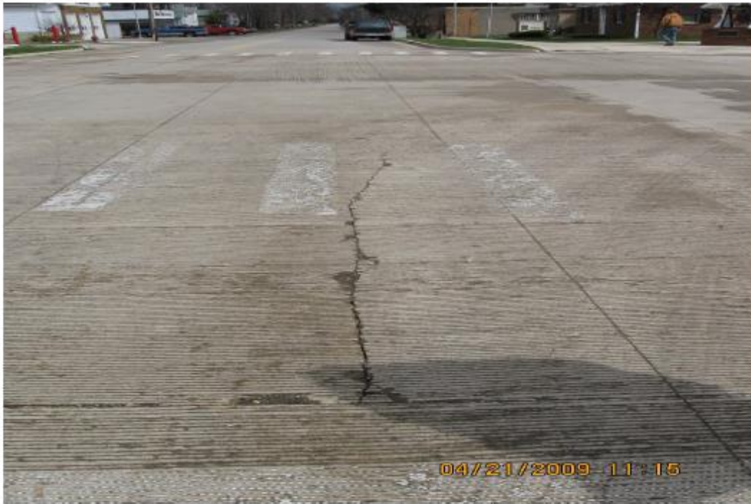
South Leg of M-99/Maple additional Long. crack
