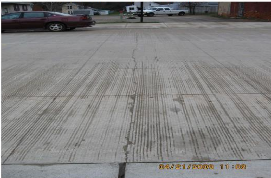
Transverse crack 225' north of Pearl St. across entire roadbed
