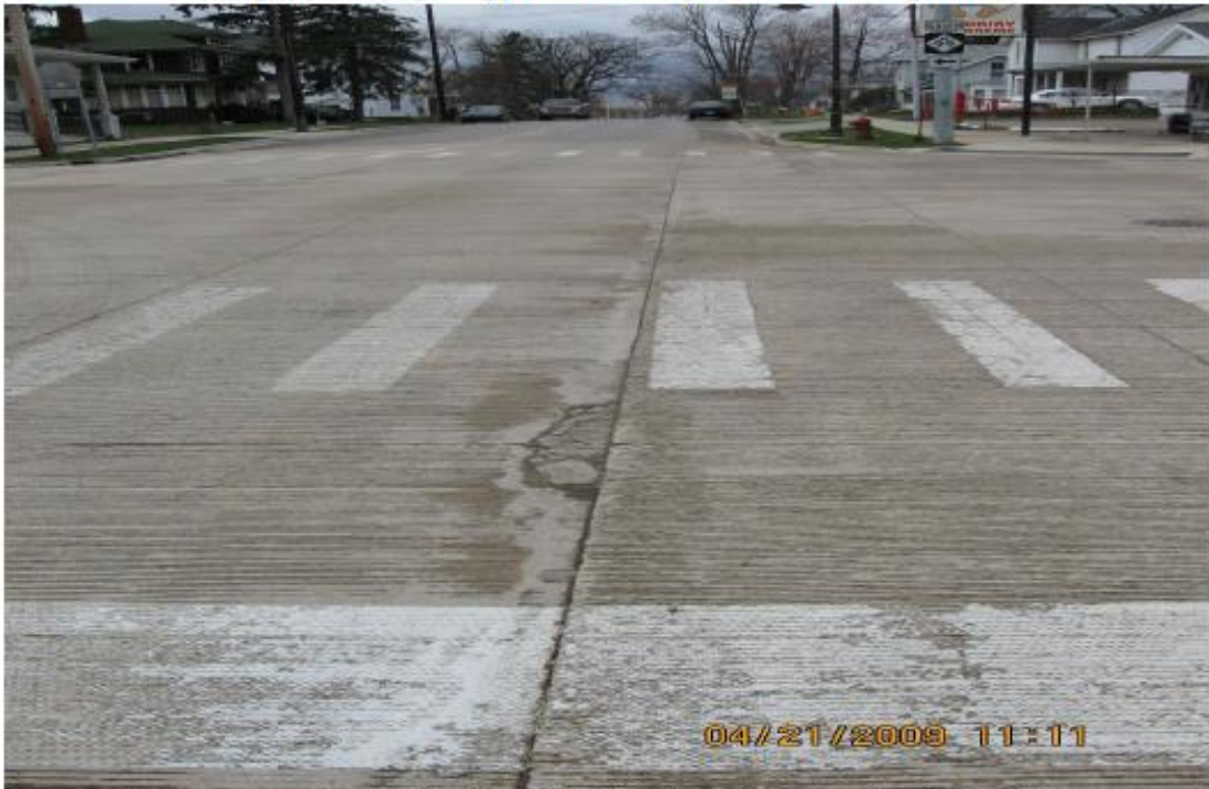
Transverse Crack/Spall at Maple/M-99 intersection North leg
