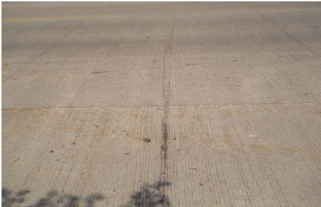
Picture #15: Transverse crack (3 slabs).
