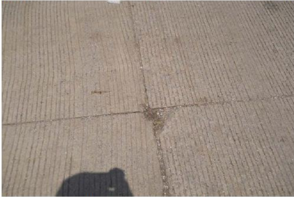
Picture #7: Corner spall.
