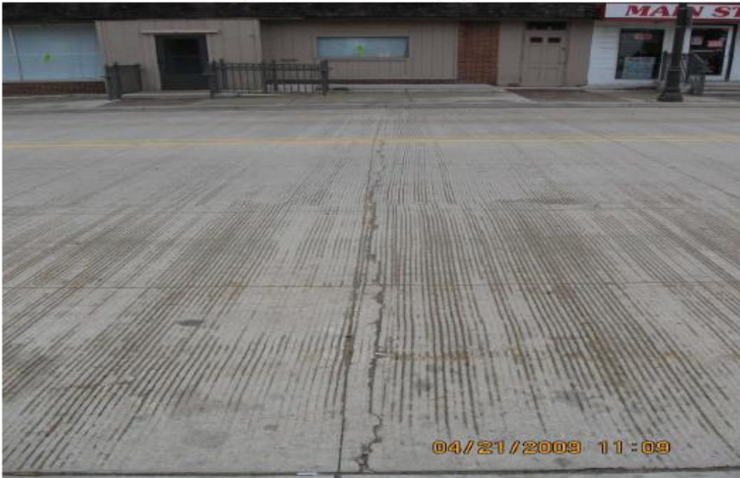
Transverse crack 150' south of Maple
