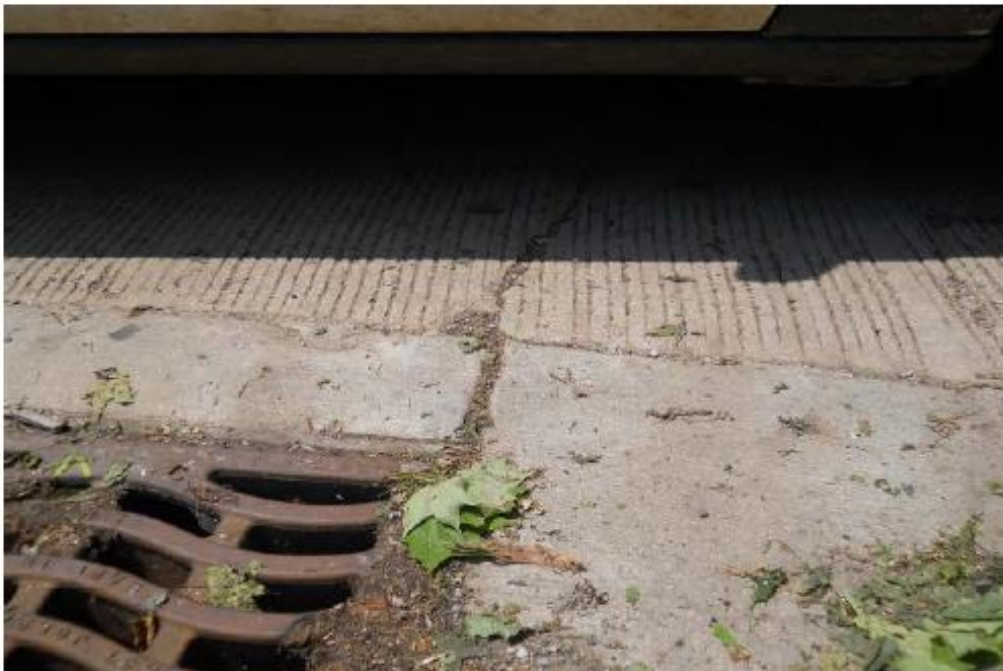
Picture #4: Transverse cracking to edge of panel.
