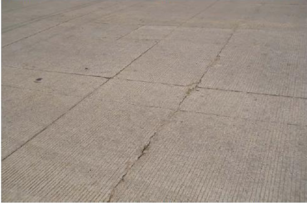
Picture #17: Mid-panel transverse crack.
