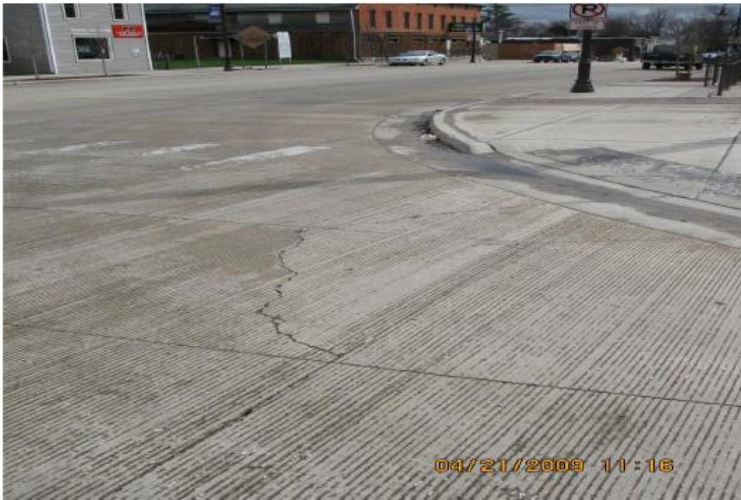
Corner crack/Transverse crack in SE radius of M-99 and Maple
