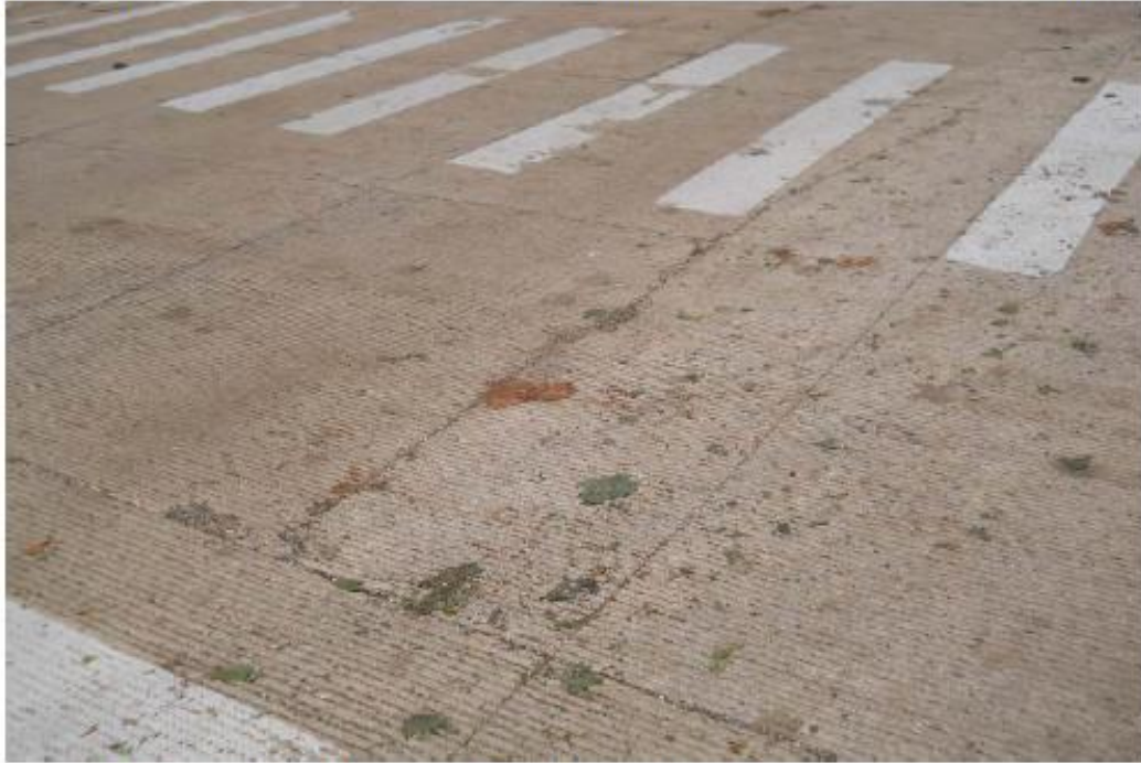
Picture #5: Longitudinal cracking (three panels).
