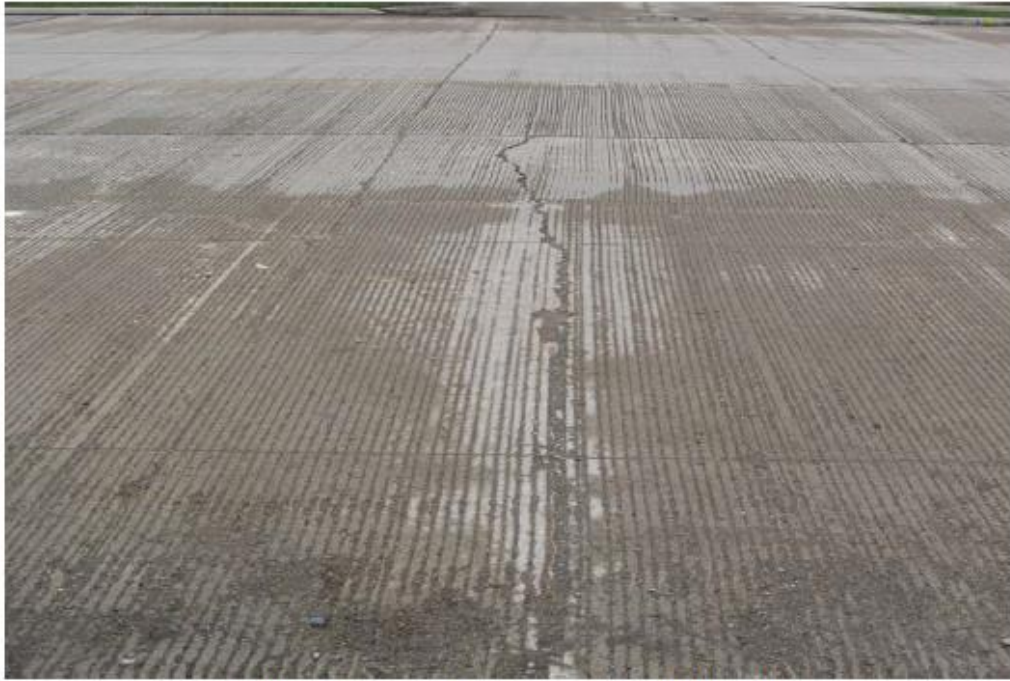
M-99 Transverse Cracking near POE, NB-1
