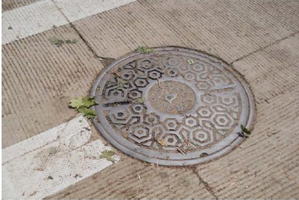
Picture #1: Spall and cracking around MH.
