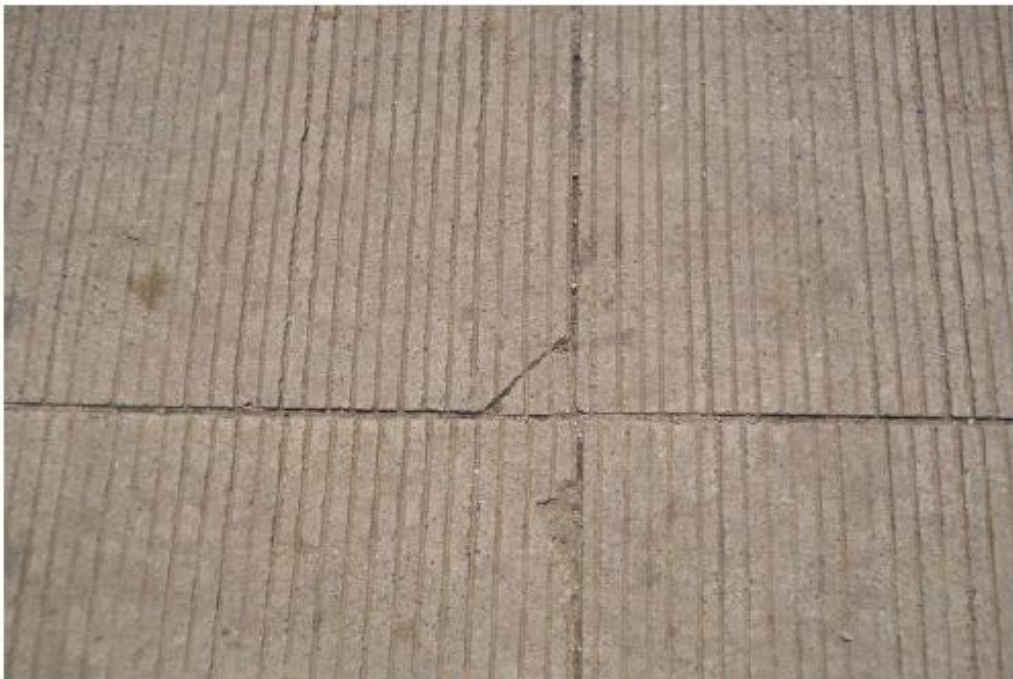
Picture #14: Corner crack.
