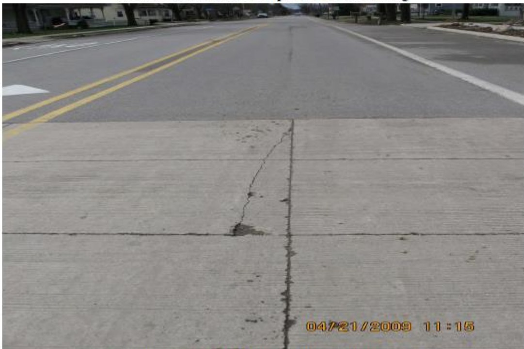
South leg of M-99/Maple, Longitudinal crack
