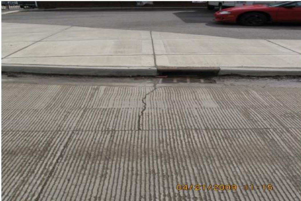
South leg of M-99/Maple, transverse crack
