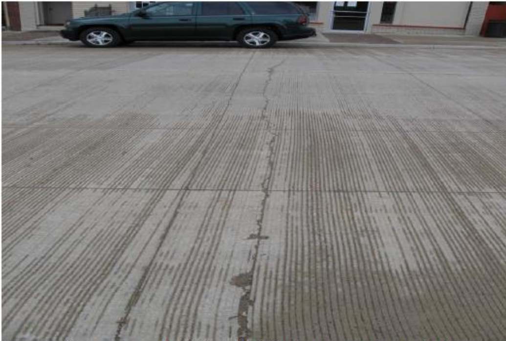
Transverse crack 130' north of Pearl across entire roadbed
