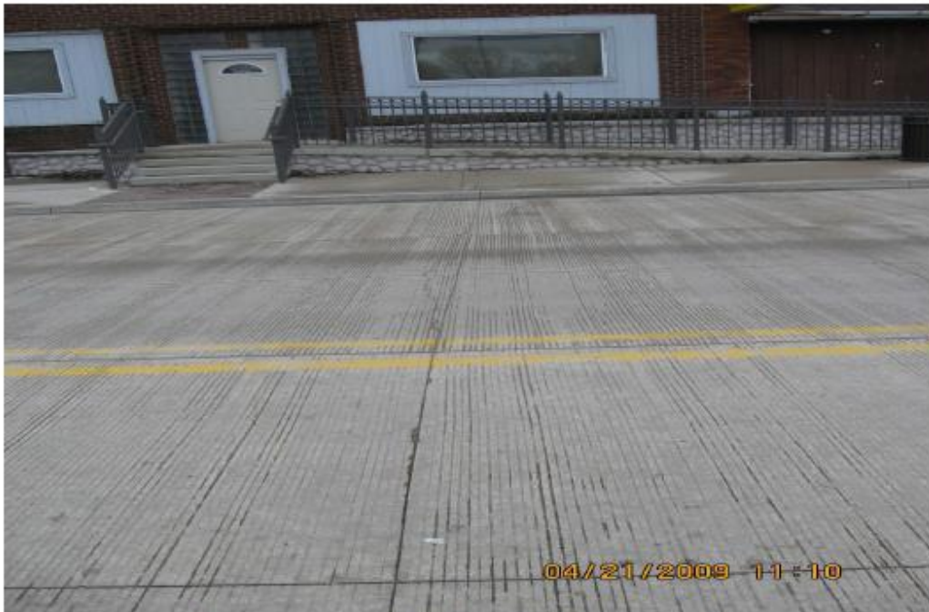
Transverse crack 200' south of Maple in SB-1
