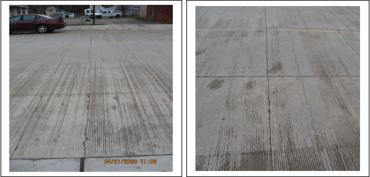
Figure 8. Transverse and Corner Cracks on M-99 from MDOT Warranty Report SWAD 2870 (2009)
