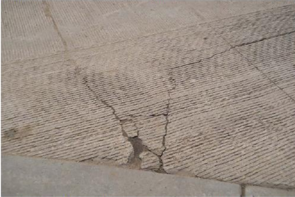
Picture #19: Cracking/spalling near curb and gutter.
