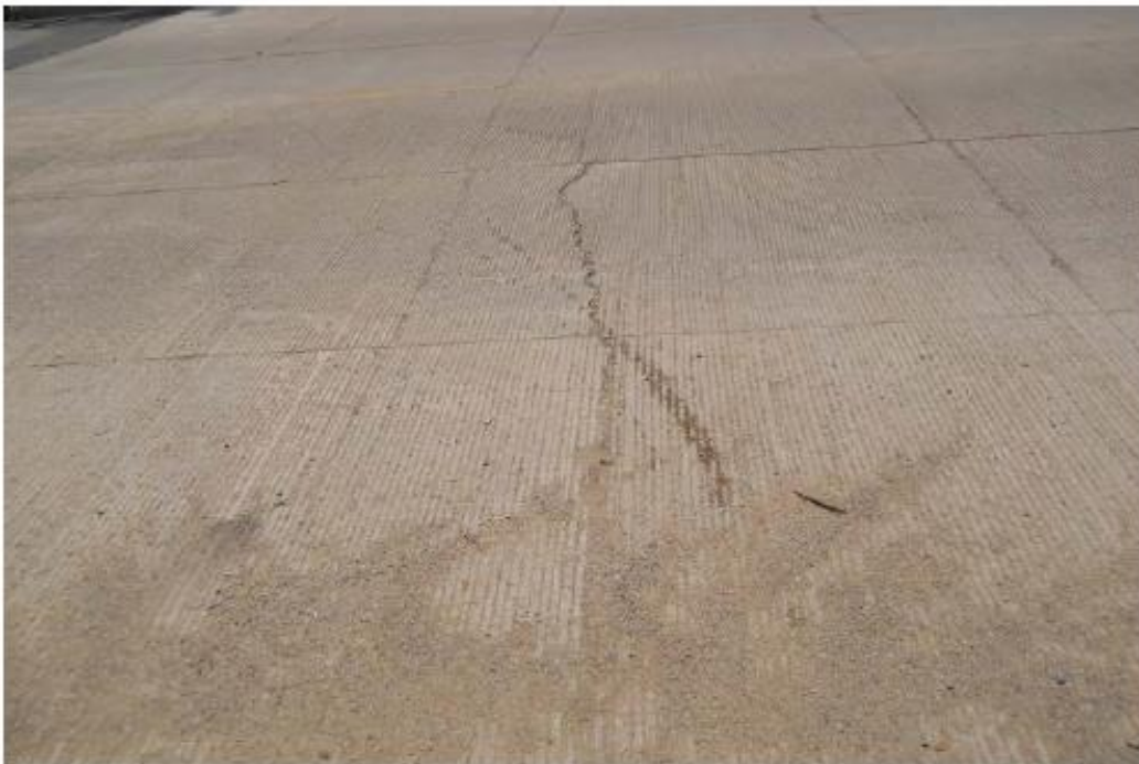
Picture #20: Longitudinal cracking, southbound only.
