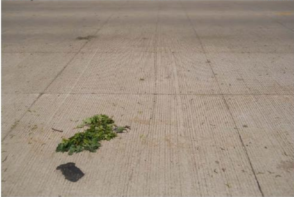
Picture #11: Mid-panel transverse crack.
