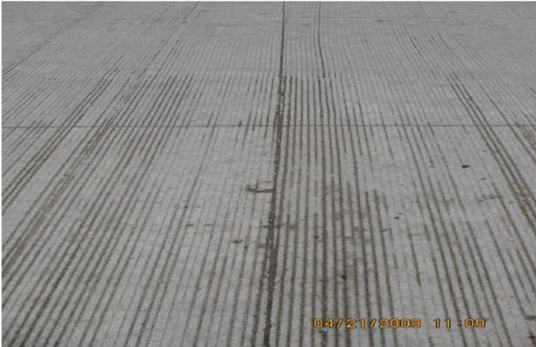
Spall 75' south of Maple SB-1
