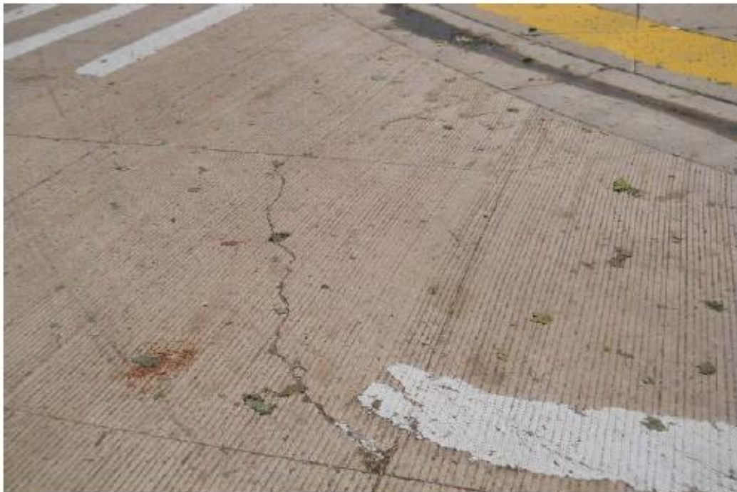
Picture #6: Cracking from curb joint through two panels.
