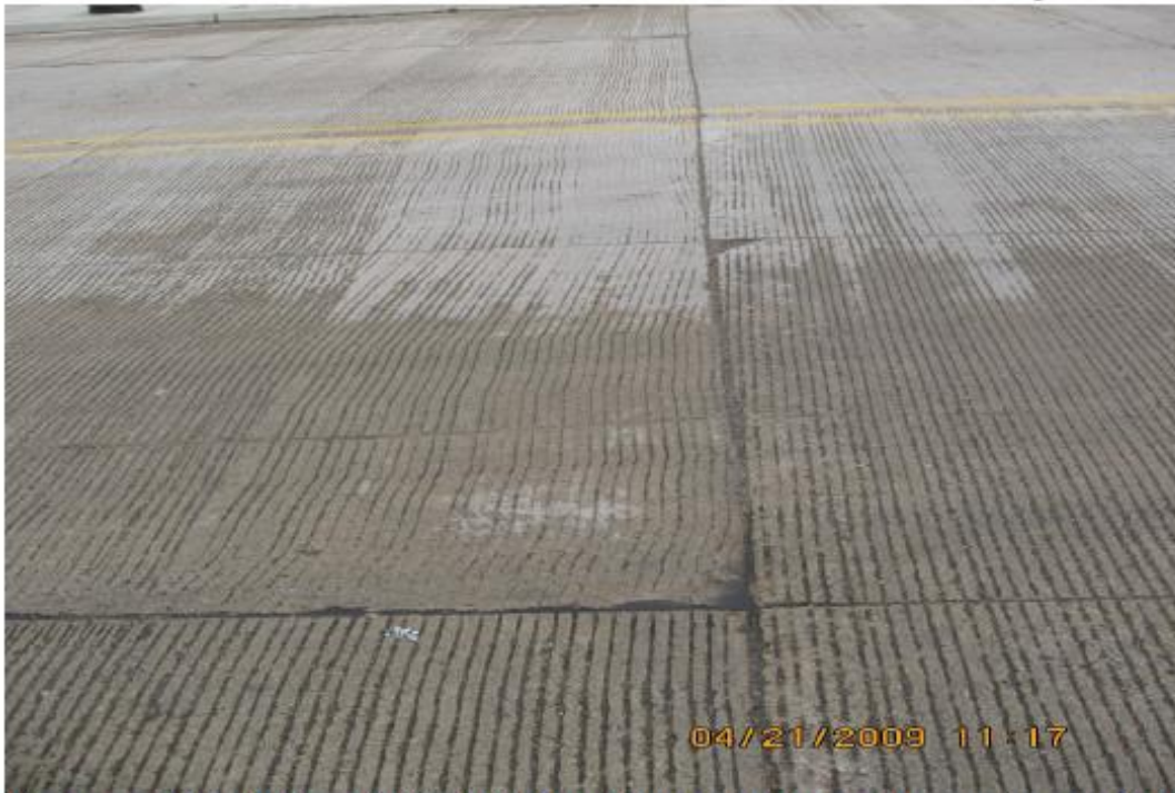
Picture of slab that has faulted with out signs of distress. East spring point of SE quad of M-99 and Maple.
