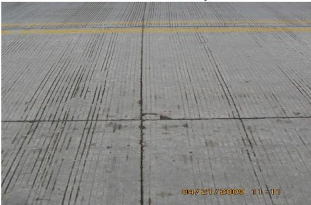
Corner crack 75' south of Maple St. in SB-1
