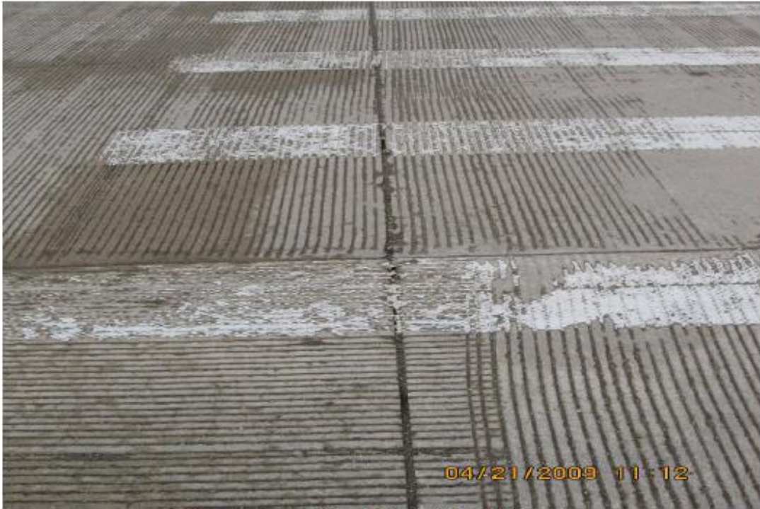
Joint sealant failure Maple/M-99 North leg
