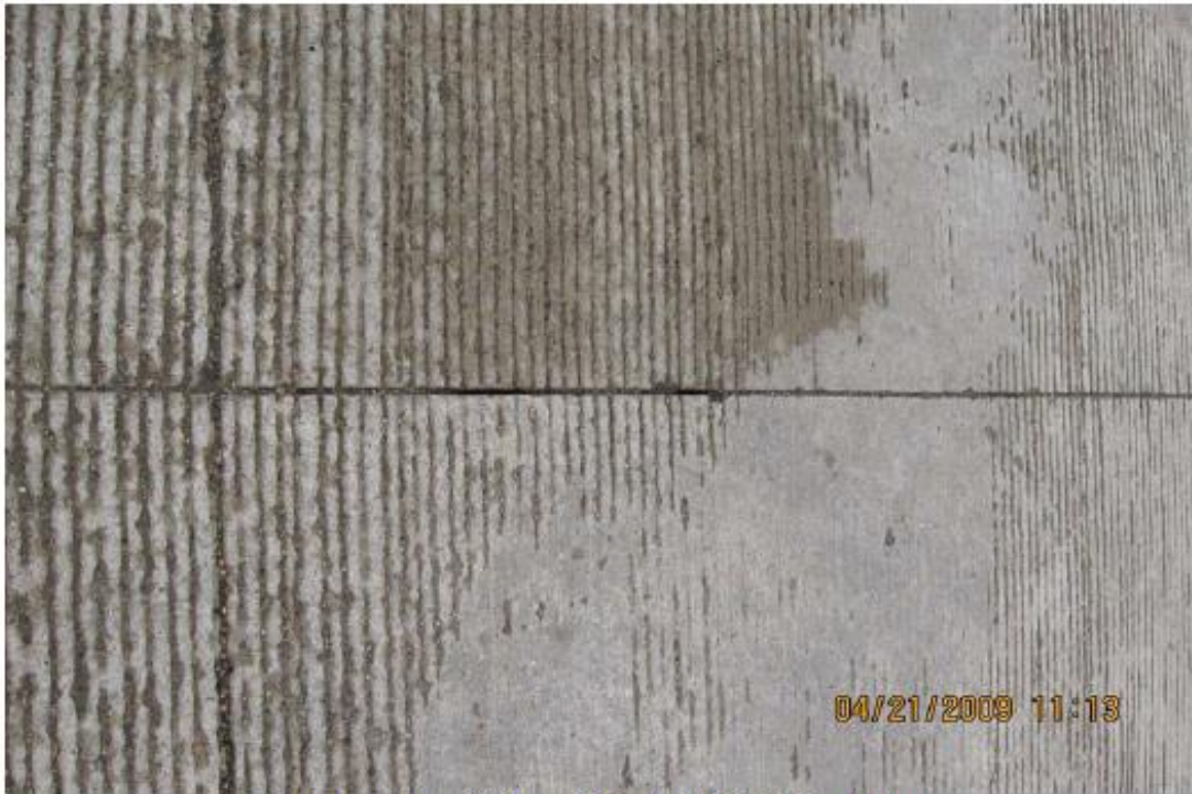
Joint sealant failure Maple/M-99 North leg
