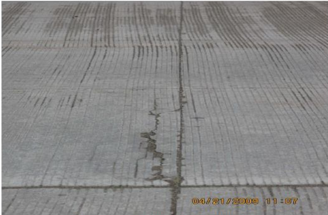
Transverse crack 180' north of Pearl St. NB-1
