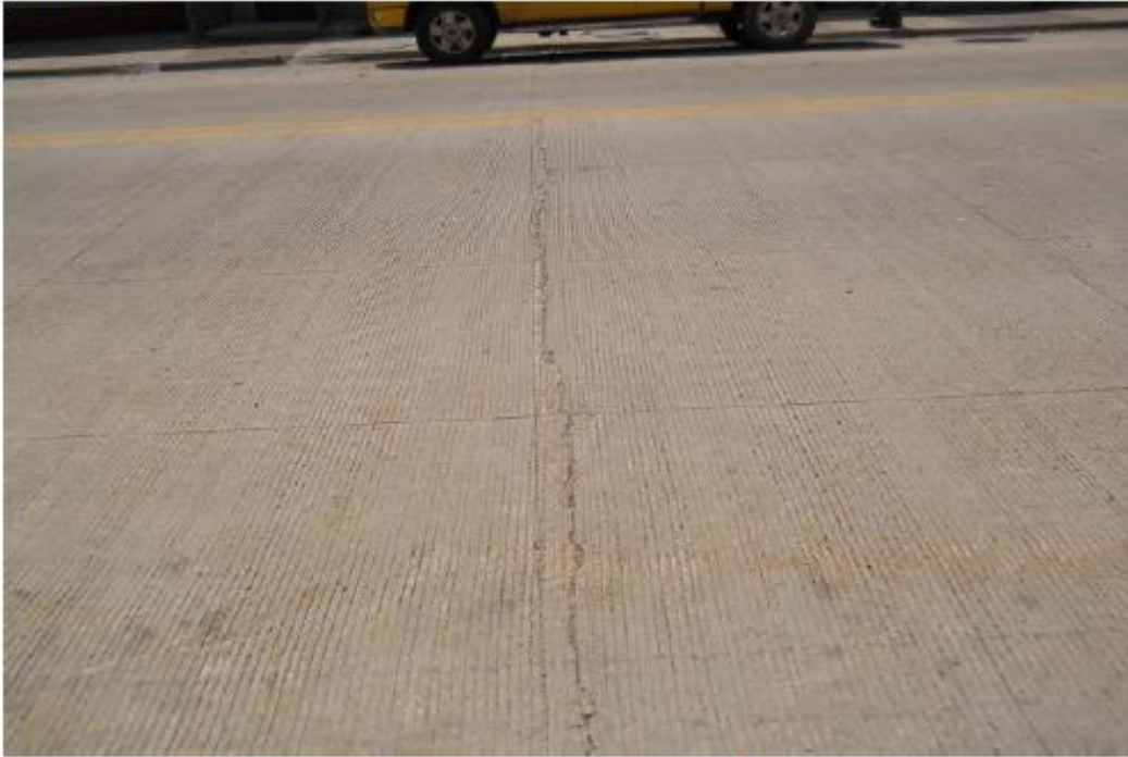
Picture #9: Transverse crack near joint.
