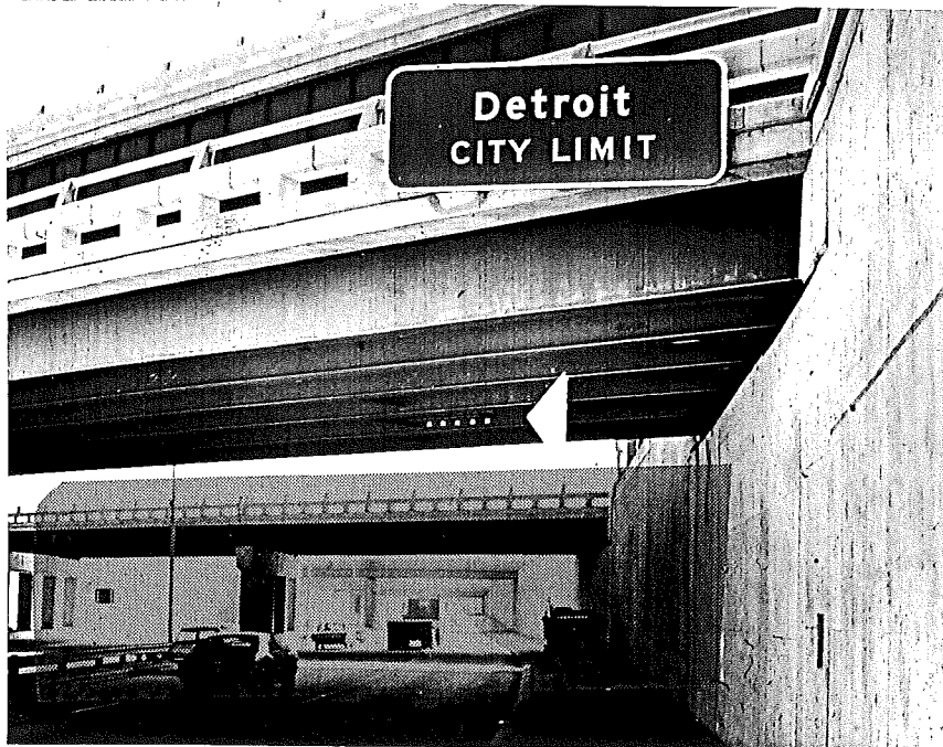
Figure 2. Location of test assemblies (indicated by arrow) over traffic lane on southbound I 696 in Detroit under Eight Mile Road.
