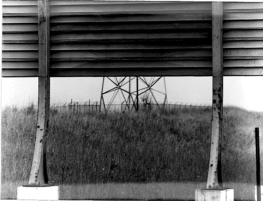
Figure 9. Relatively pronounced oxidation corrosion of steel supports of roadside signs support assembly on eastbound I 96 (legend: "New Hudson 4, Lansing 56"). Age: 2 1/2 years.
