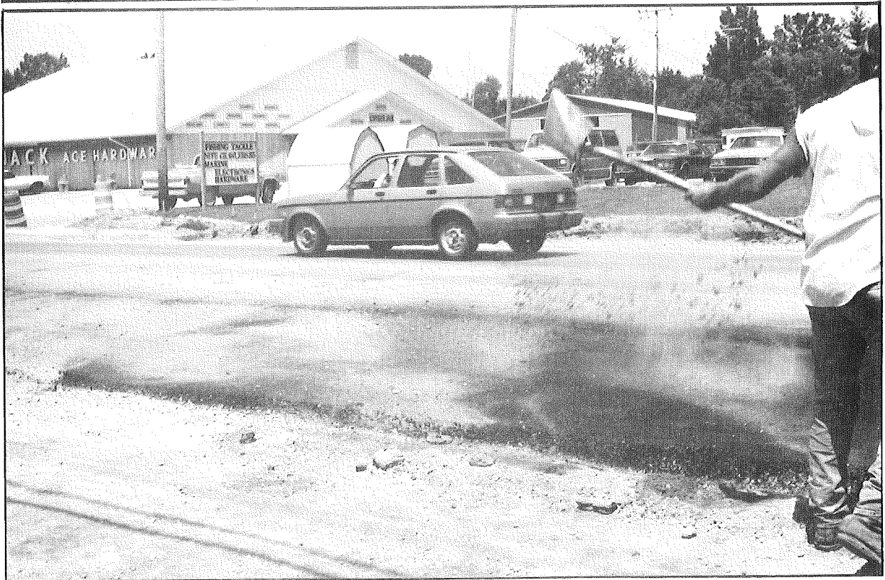
Figure 3. Bituminous curing coat being placed on LFA base course (above). Placement of a layer of soil on top of bituminous curing coat (below).
