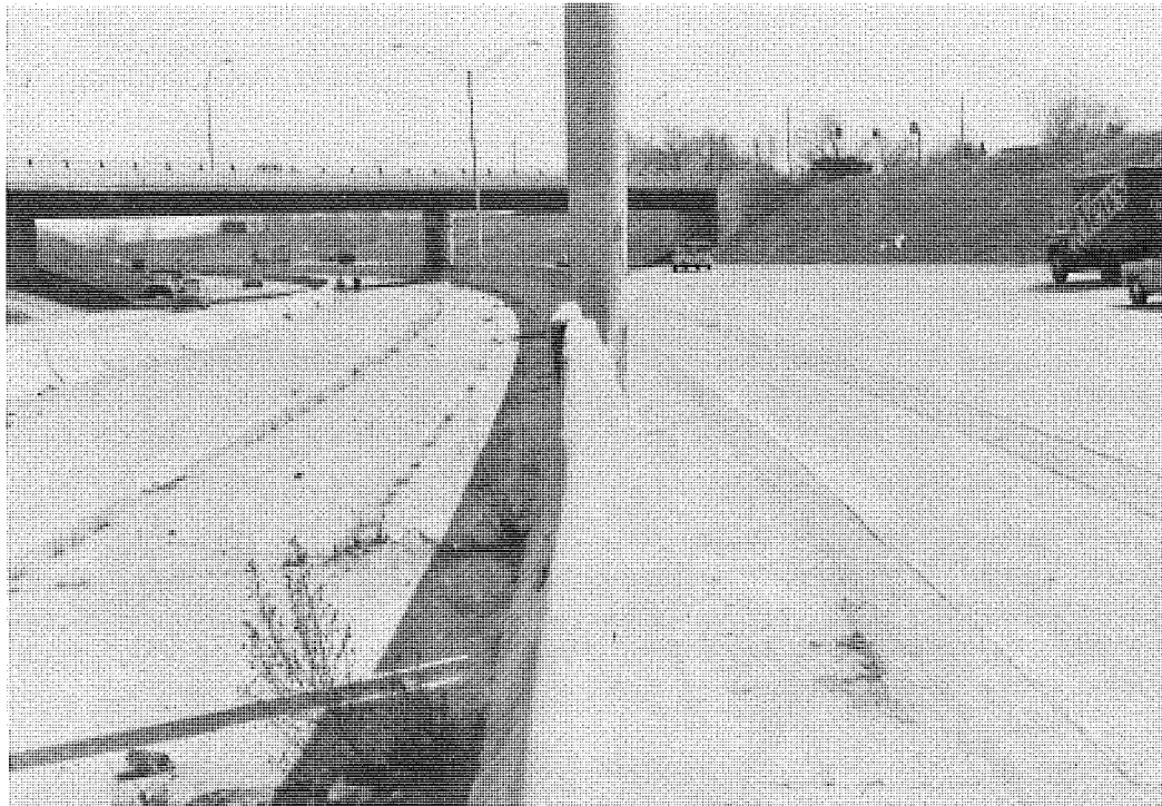
Figure 8. Section of glare screen out of alignment on I 696, spring 1983.
