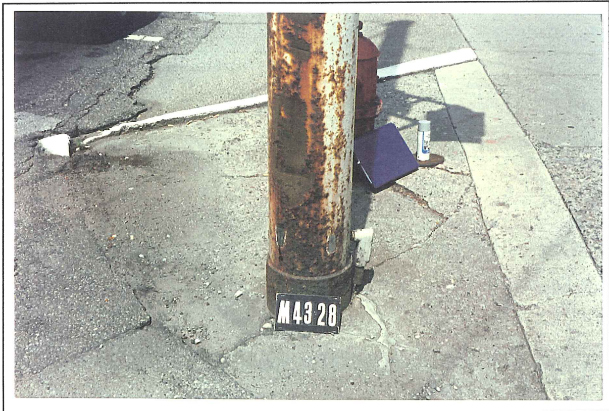
Figure 2 - Typical Painted Steel Strain Pole with Buried Foundation
