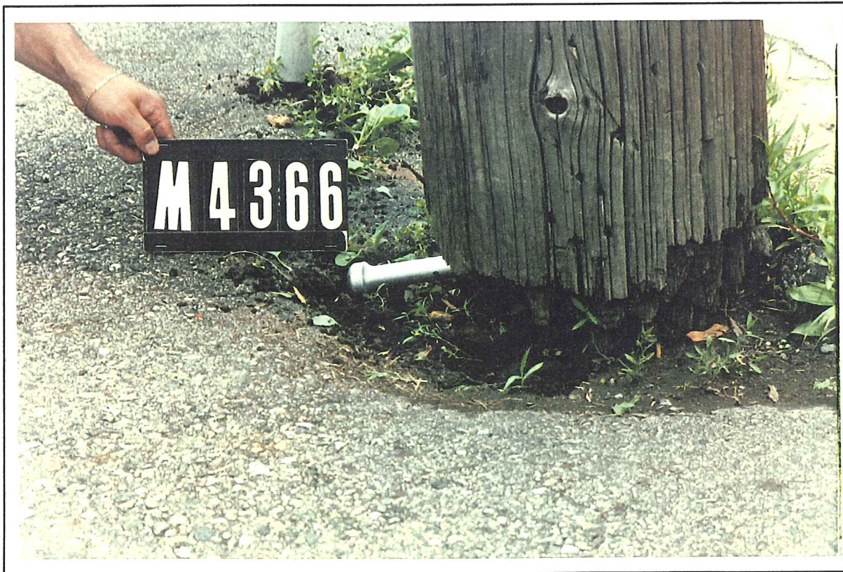
Figure 11 - Wood Strain Pole with Severe Section Loss
