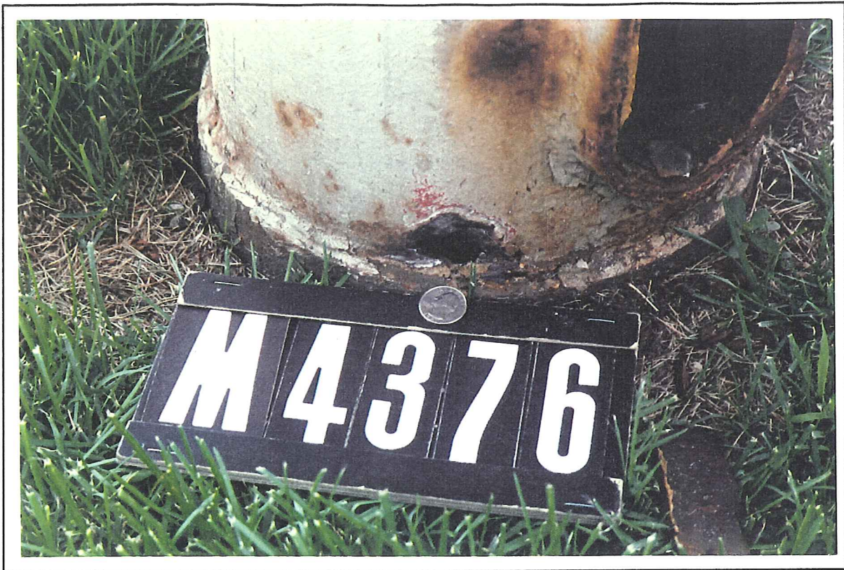
Figure 10 - Heavily Corroded Painted Steel Strain Pole
