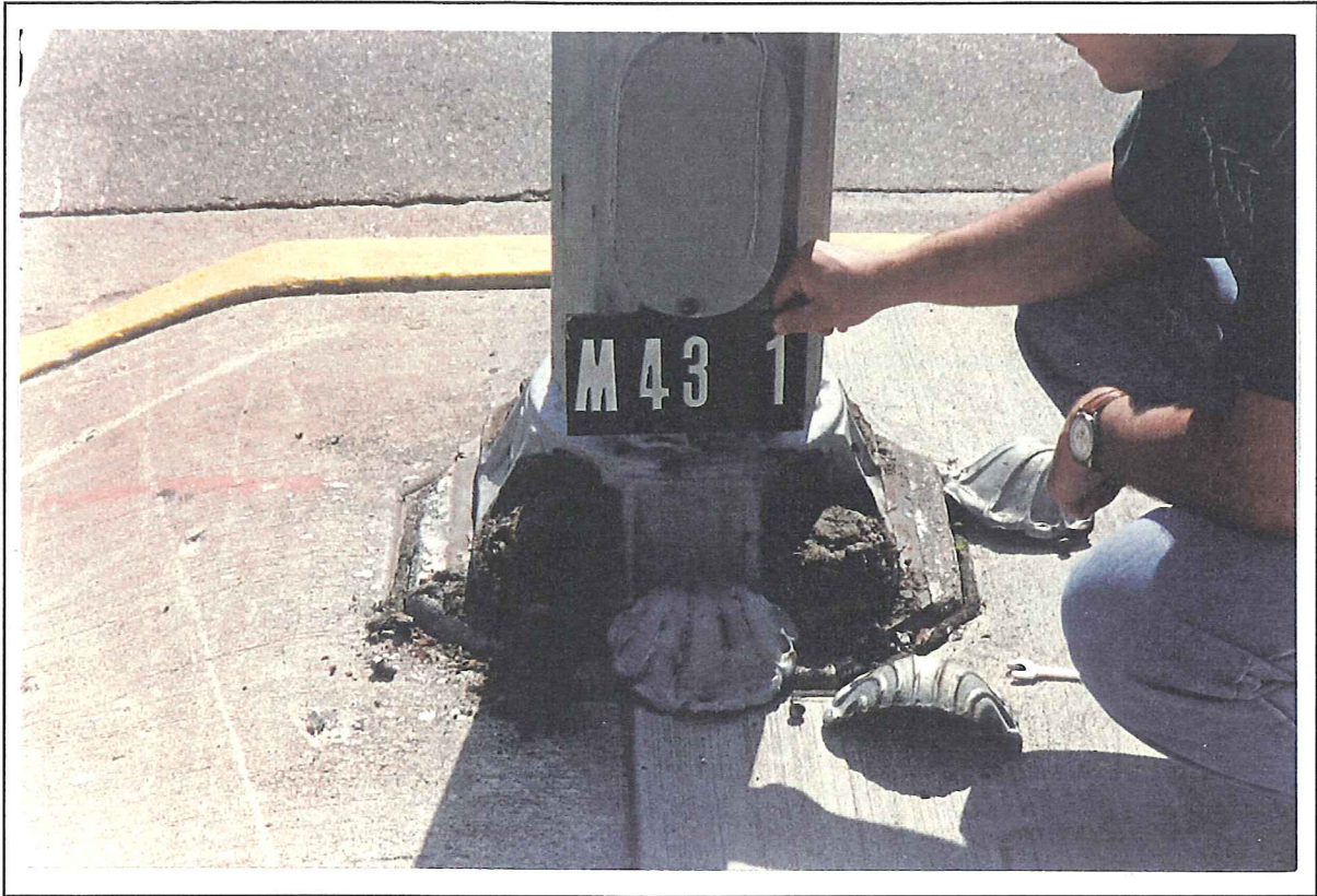
Figure 12 - Corrosion of Anchor Bolts and Nuts Accelerated by the Use of Nut/Bolt Covers
