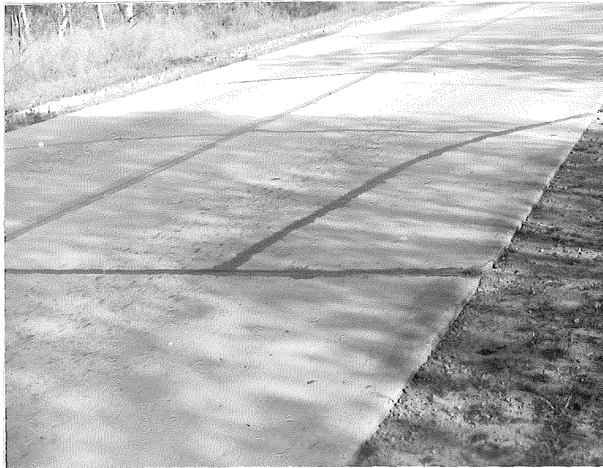
Figure 4. Corner break and transverse crack in patch right lane at Station 212+00 looking north.
