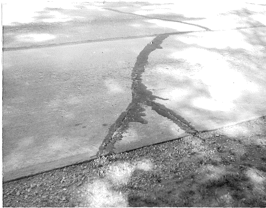
Figure 3. Cracking of new patch at Station 419+00 showing subsequent breaking out and faulting of section at slab edge.
