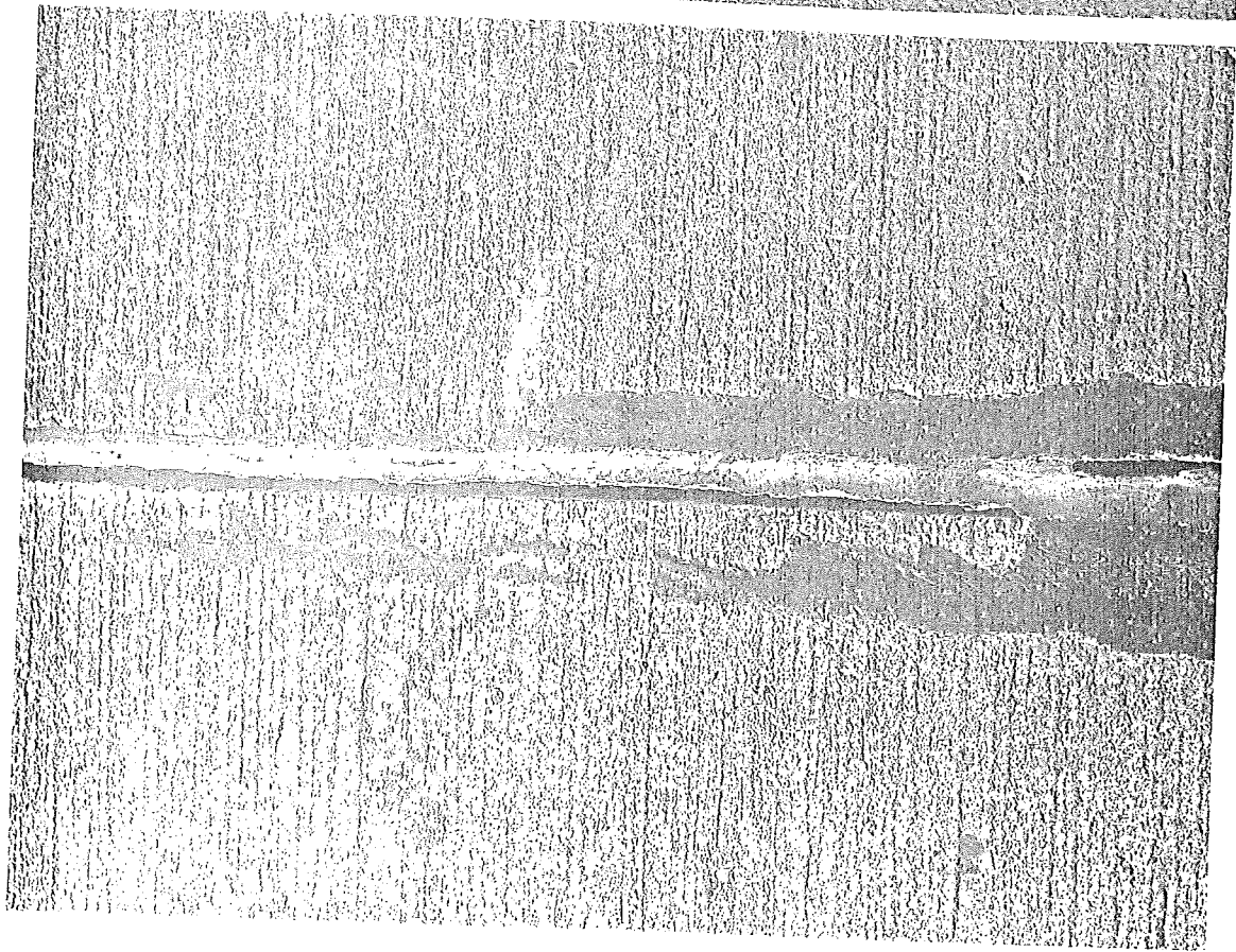
Figure A34. Joint seal adhesion failure. A bond failure between joint seal and the face of the joint seal groove.
