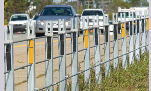
This straight-line design is one of five high-tension cable barrier systems approved for use in Michigan.
