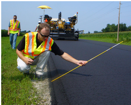
An engineer measures a fresh 30-degree Safety Edge during construction. (Courtesy of FHWA.)
