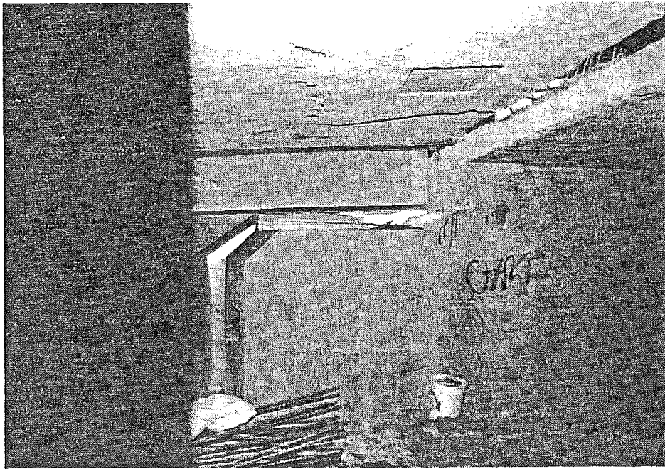
FIGURE 7. Expansion joint bearing. Note cracking of top slab
