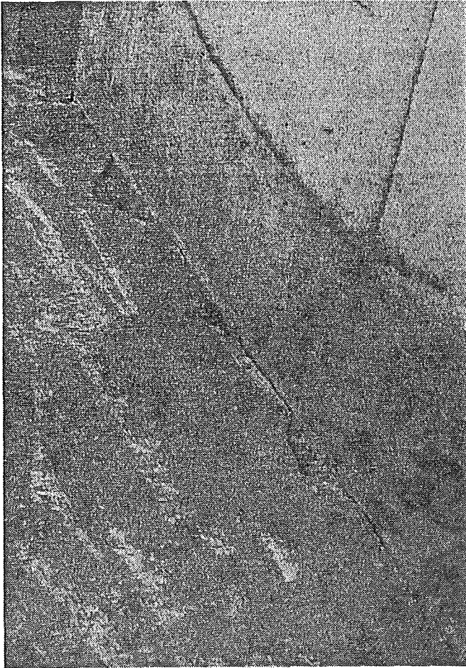
FIGURE 10. Footing spall along face of column Pier 11N.
