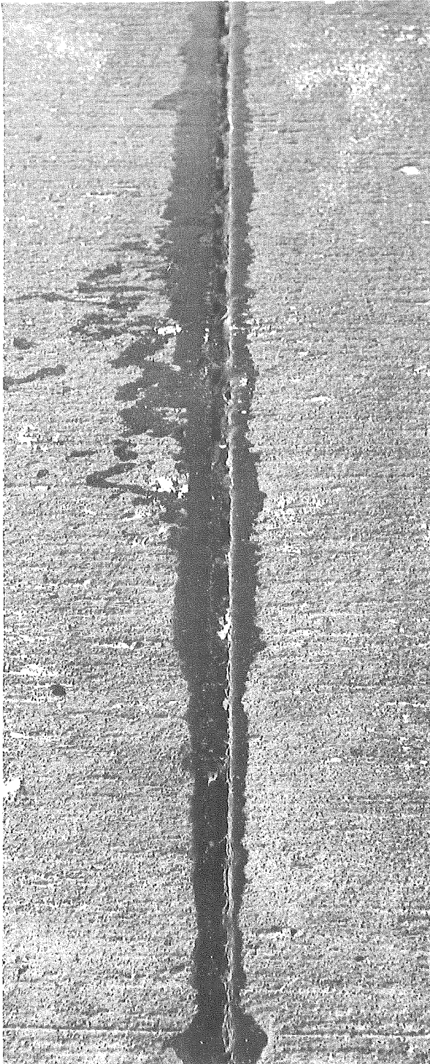
Figure 26. Pronounced adhesion and cohesion failure of hot-pour joint seal (westbound traffic lane, Sta. 649+00, Project EBACI 33083A, C1).
