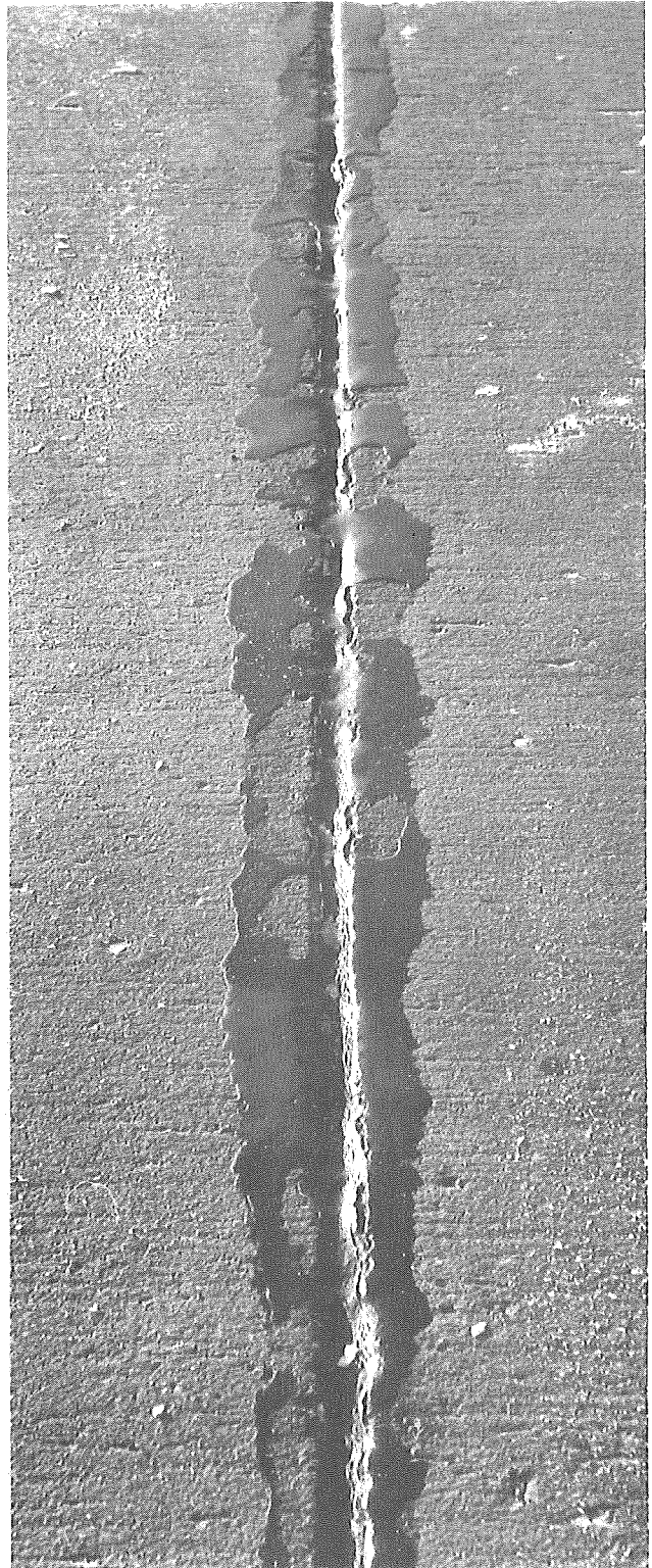
Figure 27. Some cohesion failure of hot-pour joint seal (westbound traffic lane, Sta. 553+08, Project EBACI 23151A, C1).
