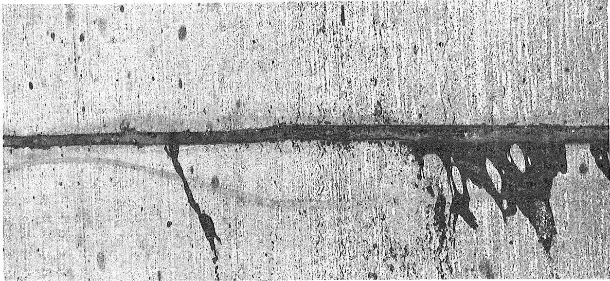
Figure 13. Typical severe adhesion failure with embedded dirt (Project BI 50112A, C1, Sta. 798+02 NB).
