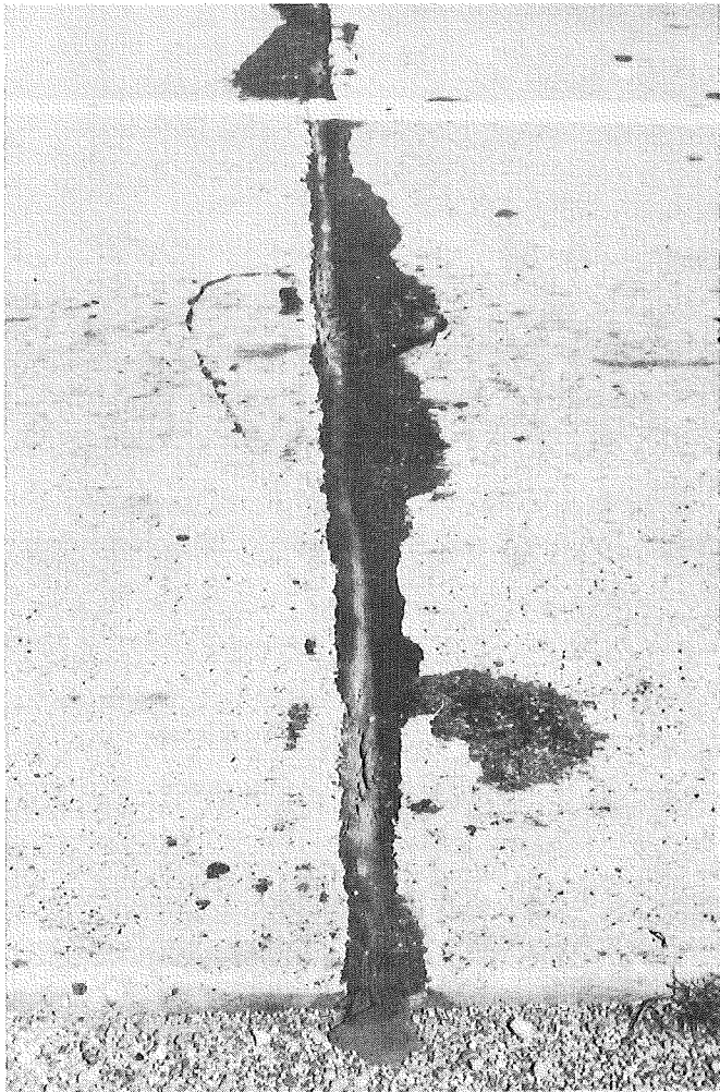
FIGURE 24. TYPICAL OF SURFACE CRACKING AND WRINKLING OF BRAND C AT 3 YEARS. SEAL STILL INTACT.
