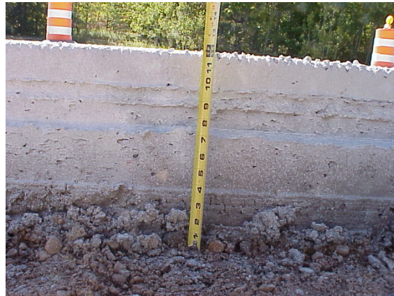
Figure 11. Area where the concrete overlay was twelve inches thick. This was at the outside shoulder joint.
