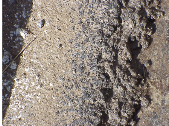
Figure 9. Voids in the separator layer are plugged with construction debris.
