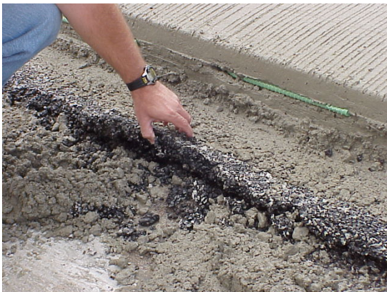
Figure 7. Loose asphalt separator layer. Note embedded lane tie that can not be straightened for the adjacent lane
