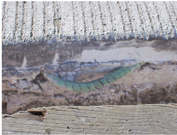
Figure 4. Tie bar embedded in the concrete. This bar can not be straightened and, therefore, is of no use.
