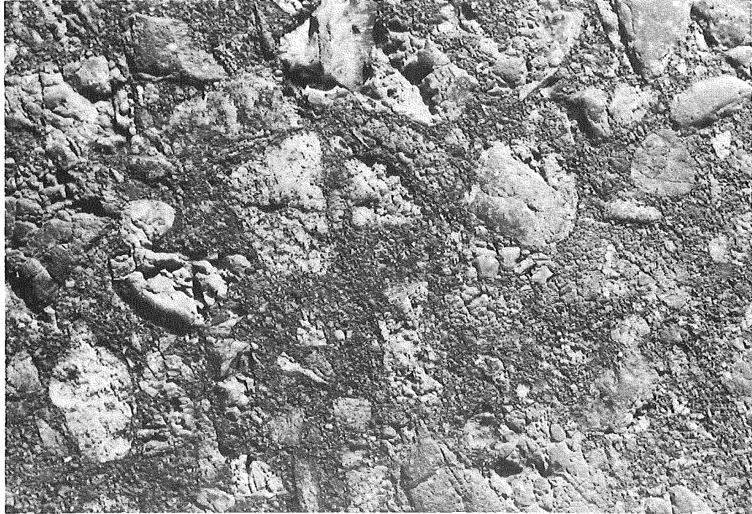
Figure 13. Bituminous concrete gravel aggregate, traffic lane, age 13 years, showing various stages of aggregate disintegration; coef. 0.55.
