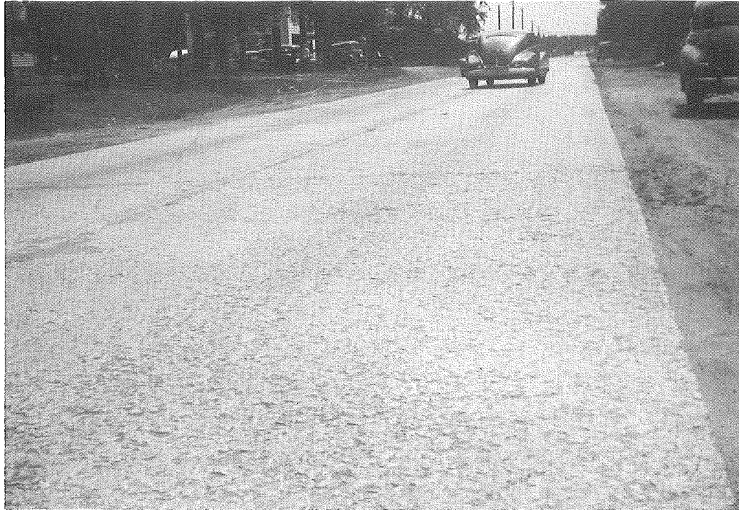
Figure 2. Typical appearance of a scaled stone sand concrete surface.
