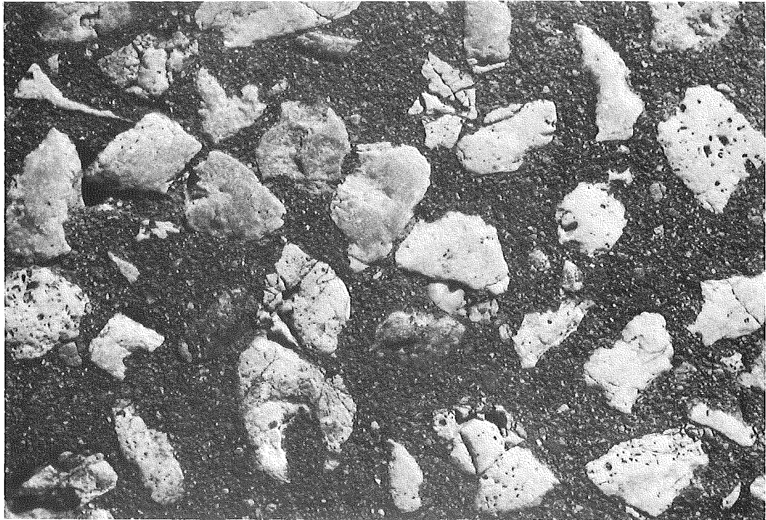
Figure 17. Bituminous concrete limestone aggregate, traffic lane, age 4 years; Coef. 0.43. Average daily traffic 2940.
