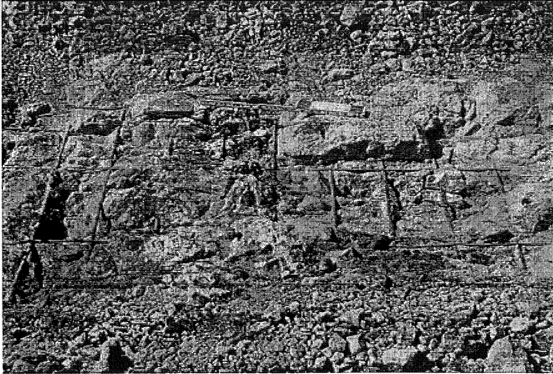
Figure B.17 US-31 SB (Elk Rapids) trench in rubble concrete (station 2+200) badger breaker
