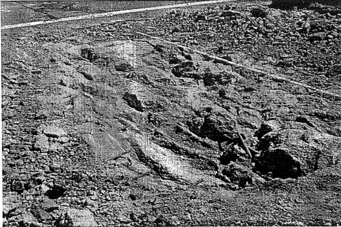
Figure B.3 M-50 EB (Dundee) trench in rubble concrete at transverse joint (station 12+000) badger breaker
