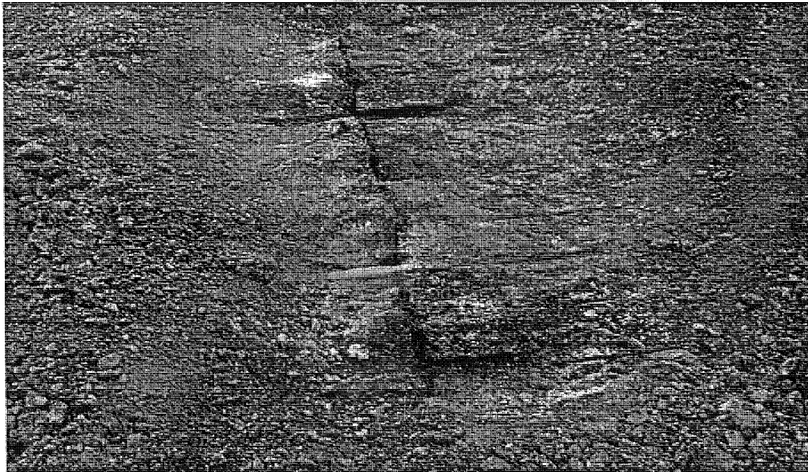
Figure B.2 US-131 SBOL (Cedar Springs) trench in rubble concrete at transverse joint resonant breaker
