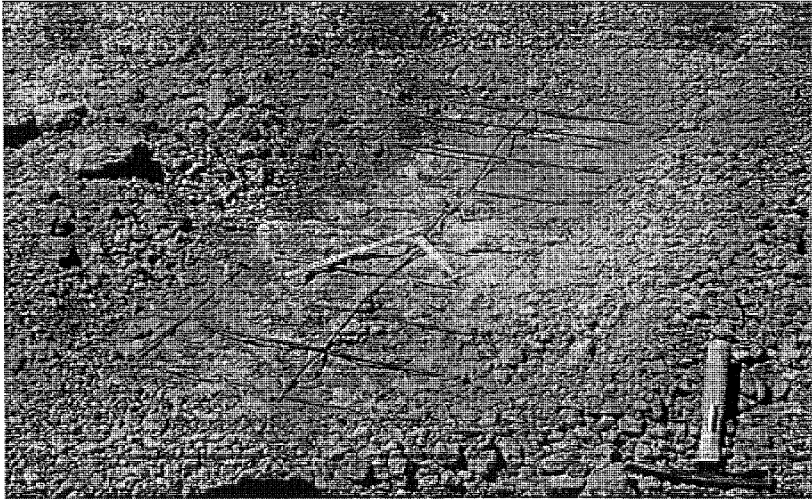
Figure B.1 US-131 SBIL (Cedar Springs) trench in rubble concrete (station 37+558.5) resonant breaker
