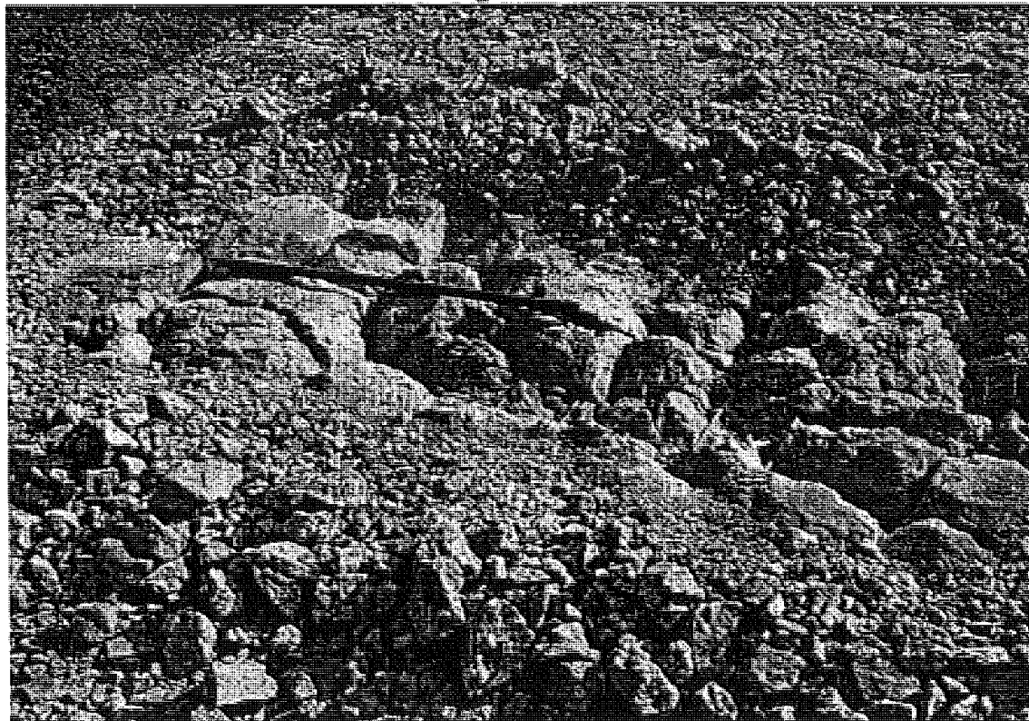
Figure B.18 US-31 SB (Elk Rapids) trench in rubble concrete (station 2+637) badger breaker
