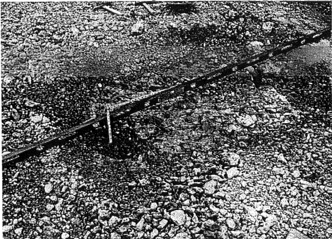
Figure B.6 US-31 SB (Honor) trench in rubble concrete (station 26+652) badger breaker
