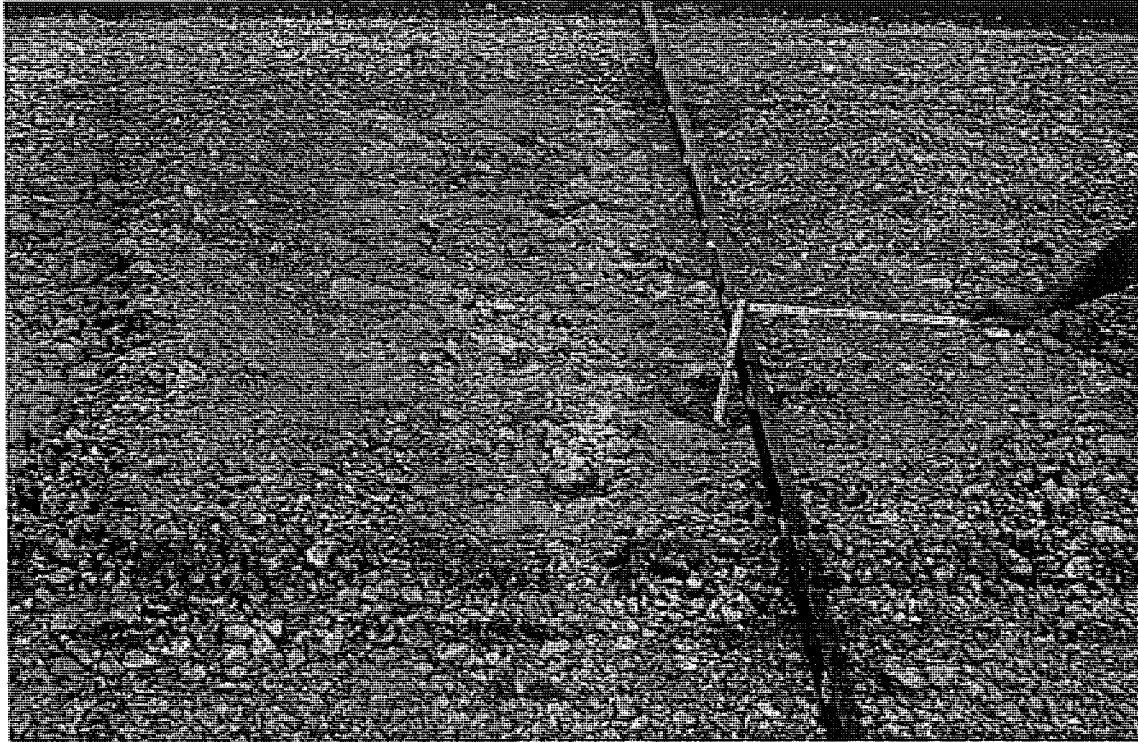
Figure B.5 US-31 SB (Honor) trench in rubble concrete (station 26+130) badger breaker
