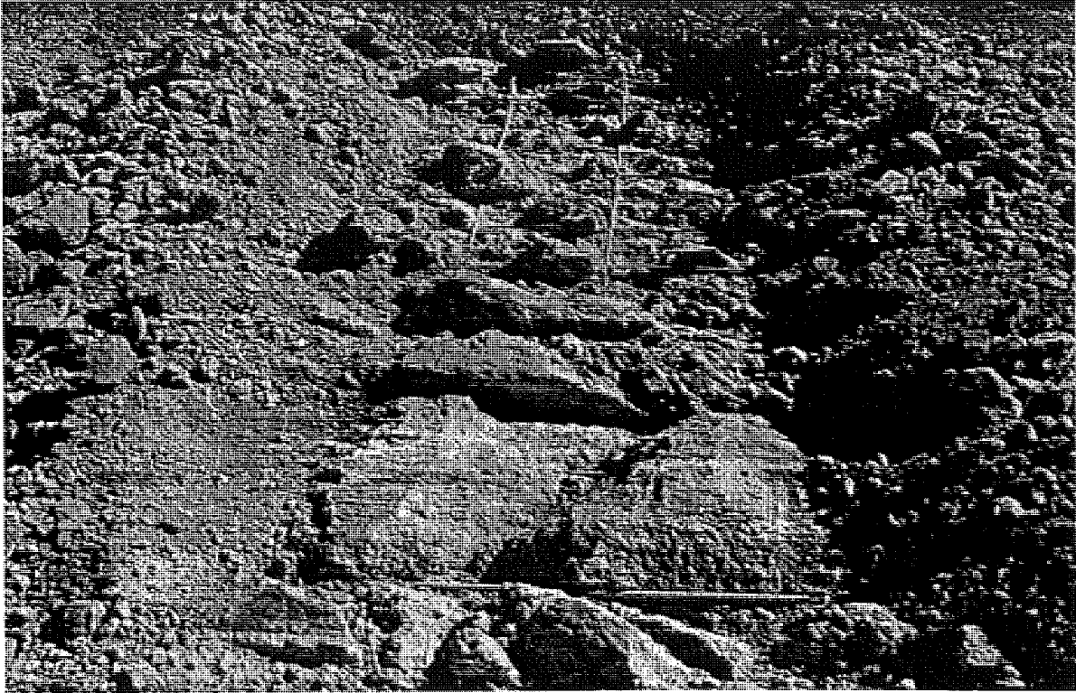
Figure B.21 US-23 SB (Alpena) trench in rubblized concrete (station 465+21) resonant breaker
