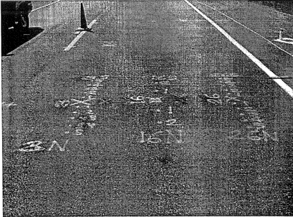
Figure C.17 Twenty four additional FWD tests and one additional core over trench area on the US-23 SB section 1 test site 1
