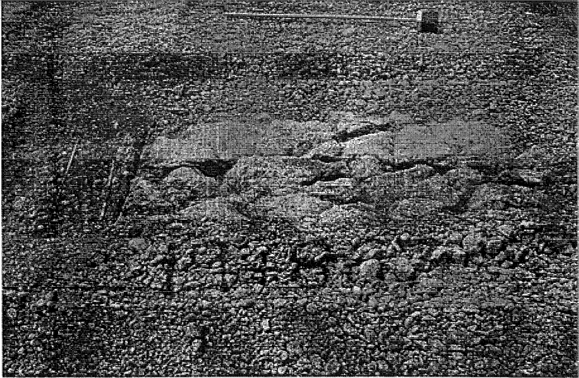
Figure B.13 US-10 EB (Evert) trench in rubblized concrete (station 19+867) badger breaker
