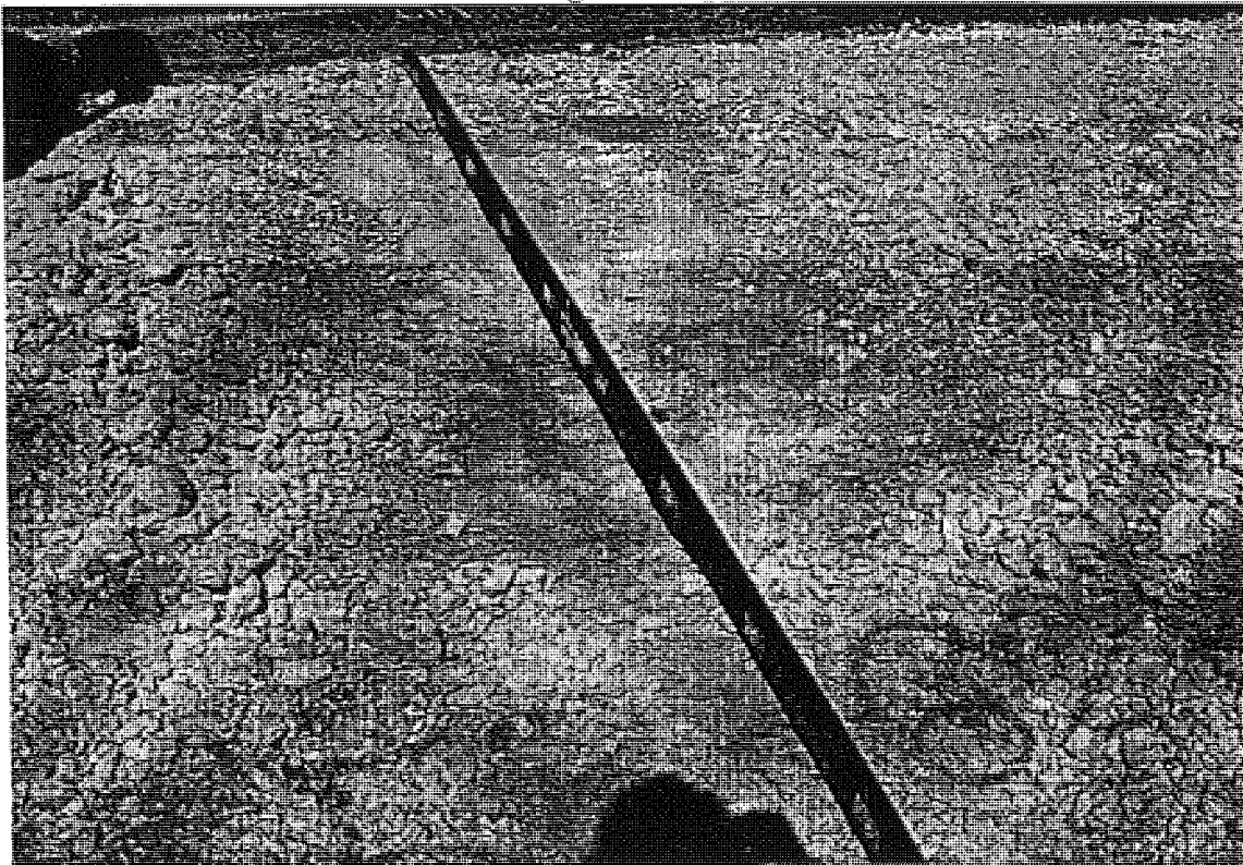
Figure B.8 M-53 NB (Almont) trench in rubble concrete (station 53+621) badger breaker
