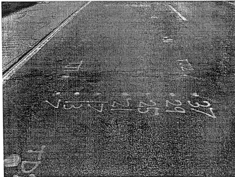
Figure C.18 Transverse joint reflective crack on US-27 SB section 2 test site 1
