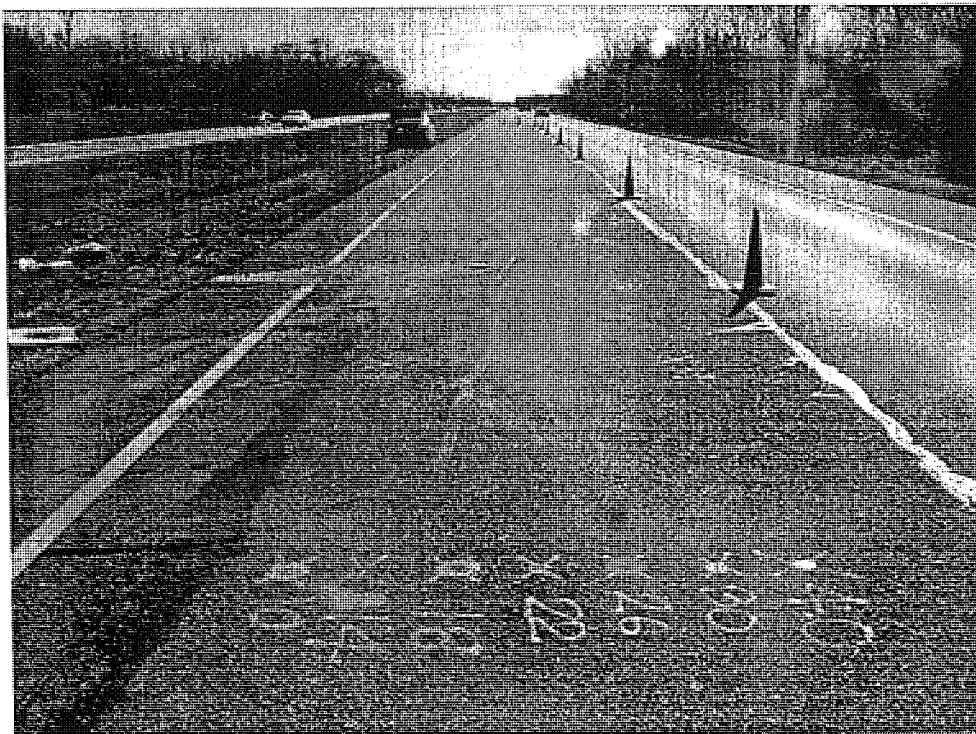
Figure C.26 M-37 SB section 6 test site 1 south of intersection between M-37 and 10 mile Rd.
