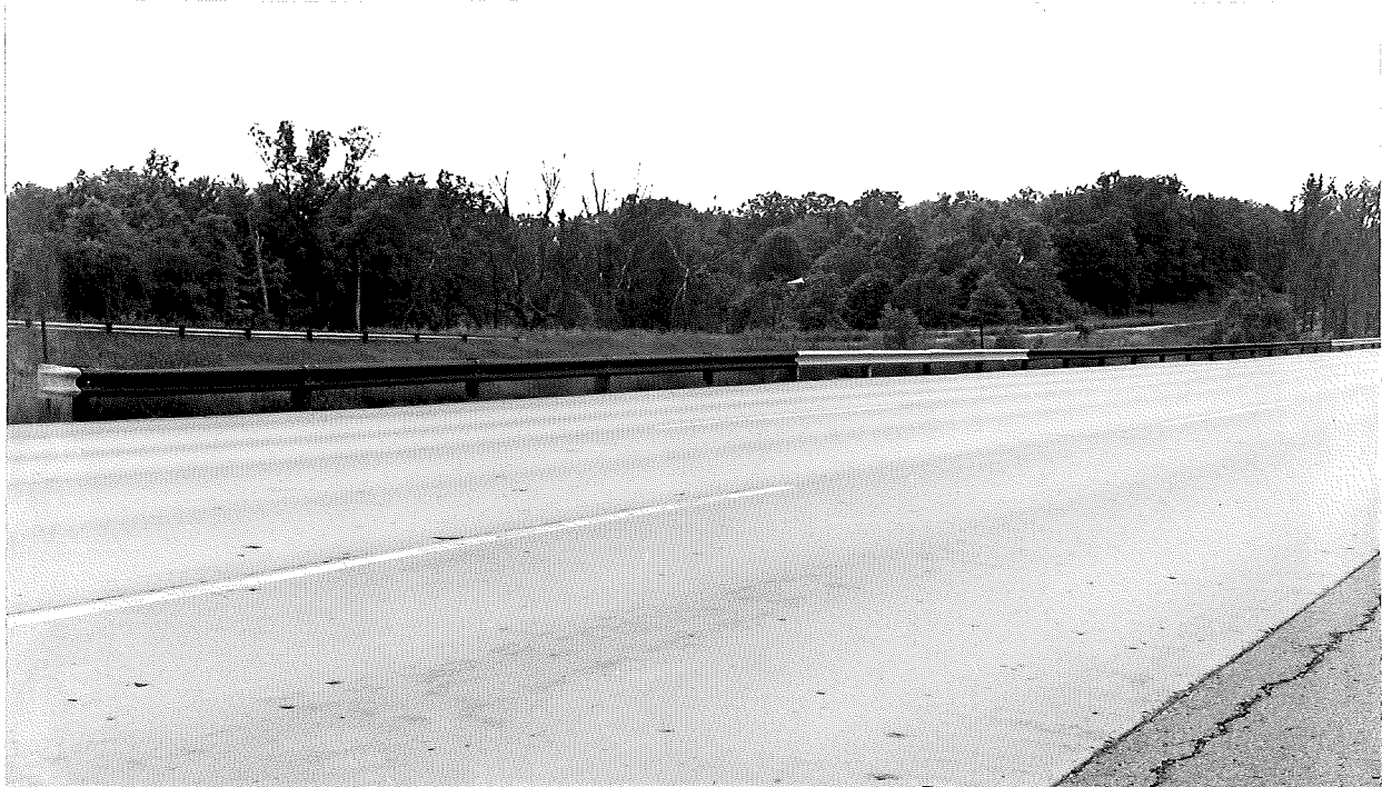
Figure 5. Daytime appearance of galvanized and unpainted alloy steel guardrails on SB I 75 N of Pontiac after about 6 yrs of service. The rails at either end are galvanized as are the four in the middle (damaged replacements).
