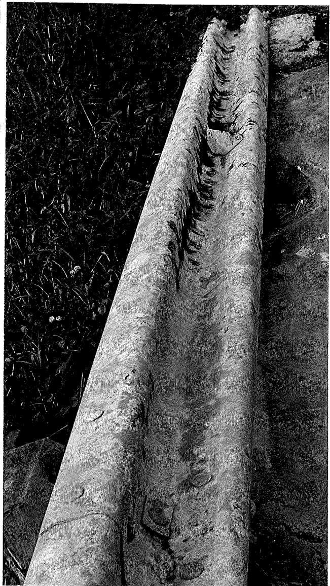
Figure 2 (right). Appearance of galvanized end-wing on I 496 in Lansing after one Winter's exposure. This was the worst railing on the project, showing much white and red rusting. Railings installed about November 1, 1968 were unable to develop protective film before Winter. The new buried type end-wing with its reflective washer is particularly susceptible since it resembles a damaged trough.
