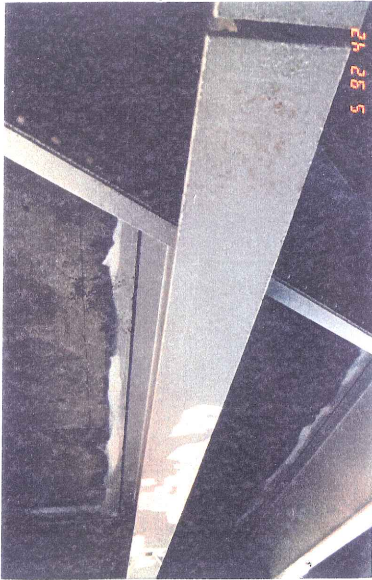
Peeling topcoat on bottom of bottom flange
