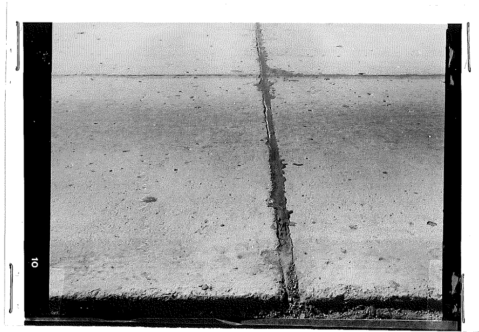
Figure 7. SOA-GRS. North half looking south. Station 183+48. Material does not bond satisfactorily. About same consistency as Hot Poured type.
