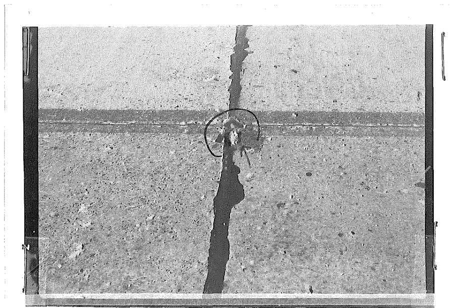
Figure 4. Paraplastic. Station 185+95. Note lack of bond where joint was not cleaned properly.
