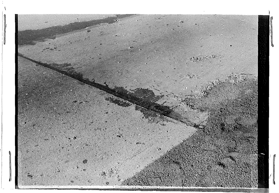
Figure 5. Oil-Revertex. South half looking north. Station 185+30. Bleeding was noticeable at edge of slab. Material too soft.
