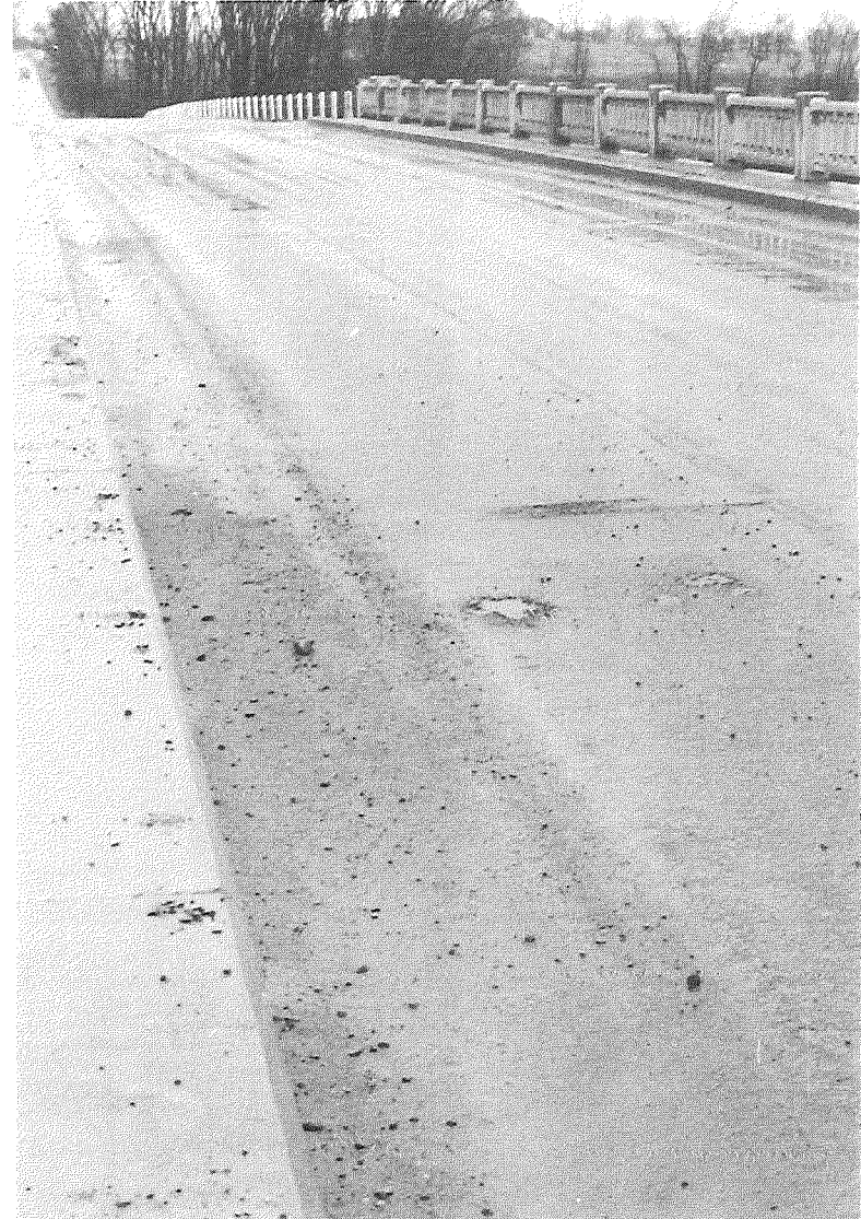
Figure 1. Dettman Road overpass, US 12 near Jackson (B9 of 38-1-14), with view of deterioration of original light wearing-surface covering (4-11-58).
