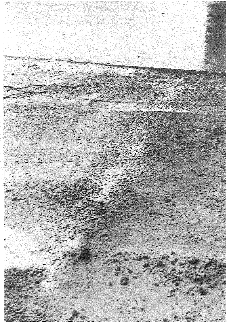
Figure 4. Undersurface seepage on Span 3 (left), with view of drip pattern on the US 12 shoulder directly beneath a longitudinal joint (right) (4-11-58).
