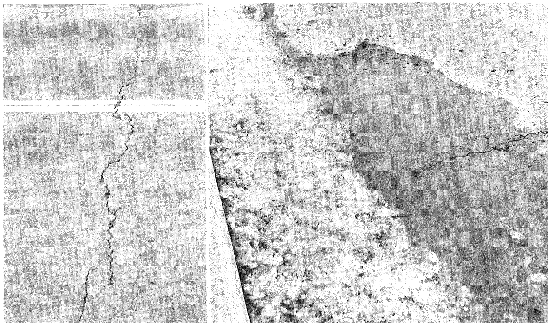
Figure 8. Reflection crack over joint (left), with view of moisture conditions at curb adjacent to same crack (2-60).
