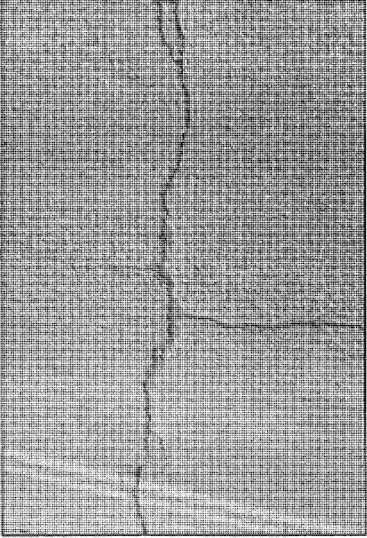
Crack that was open prior to seal coat placement that was filled with seal coat but seal coat has completely deteriorated in 1987.
