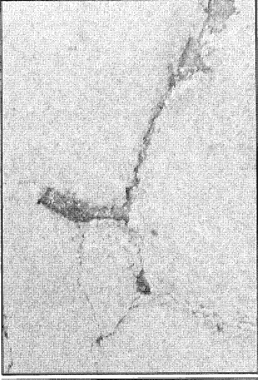
Crack that was open prior to seal coat placement that was filled with seal coat but seal coat has completely deteriorated in 1988.
