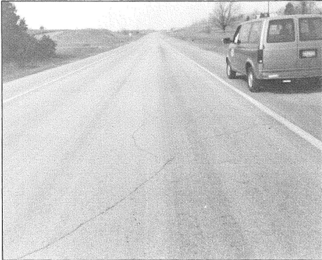
Figure 6. Scraping of center line and center of wheel paths showing loss of aggregate only.
