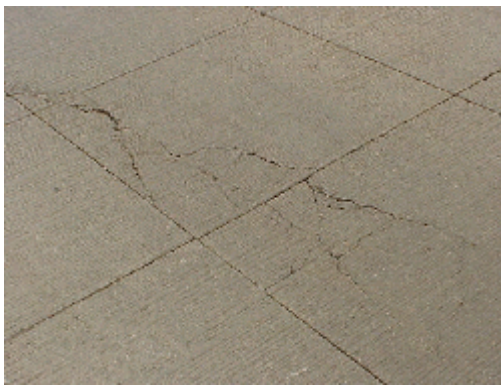
Figure 13. Another Example of Multiple Cracks.
