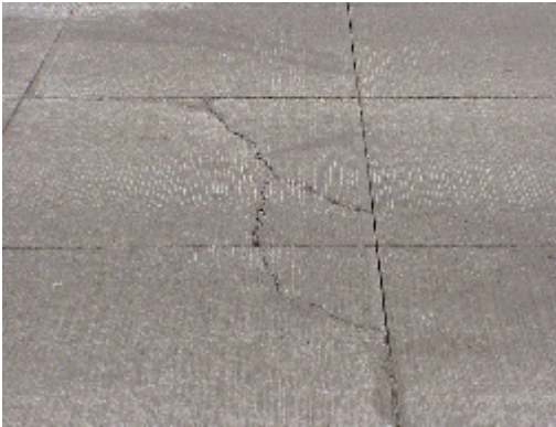
Figure 9. Example of Transverse Cracking.
