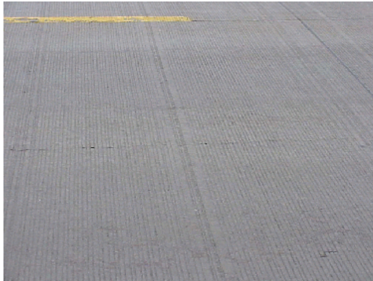
Figure 2. Initial Condition of Longitudinal Crack.
