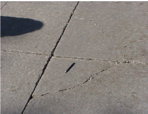
Figure 11. Example of Cracking Around the Joint Intersection.
