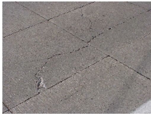
Figure 12. Example of Multiple Cracks in a Panel.
