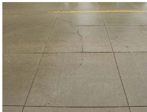
Figure 14. Another Example of Transverse Cracking.
