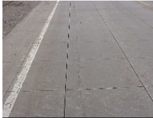
Figure 10. Example of Long Longitudinal Crack.
