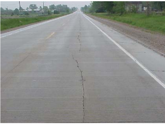
Figure 5. Looking Down the Pavement at the Long Longitudinal Crack.
