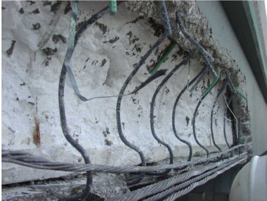
Figure 1.1-3 Damaged exterior prestressed concrete box-beam due to impact.
