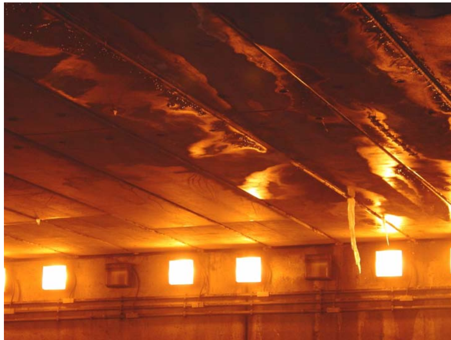
(b) Deterioration and leakage
