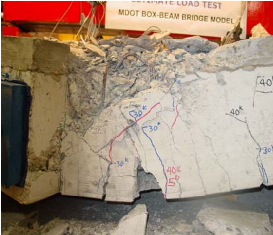
(a) Flexural cracks at mid-span
