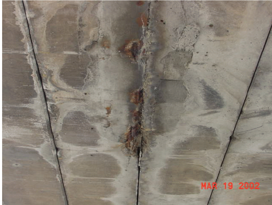
(a) Deterioration and concrete spalling
