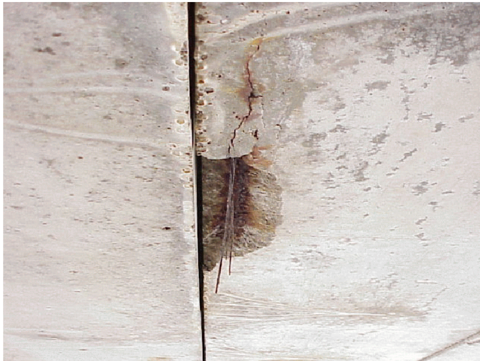
Figure 1.1-7 Corrosion of longitudinal prestressing strands.
