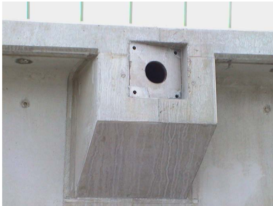
Figure 1.1-5 Close-up view of field application of transverse diaphragm for unbonded CFRP strand.
