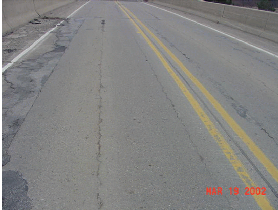
Figure 1.1-4 Longitudinal cracks in deck slab along shear-keys between box-beams.
