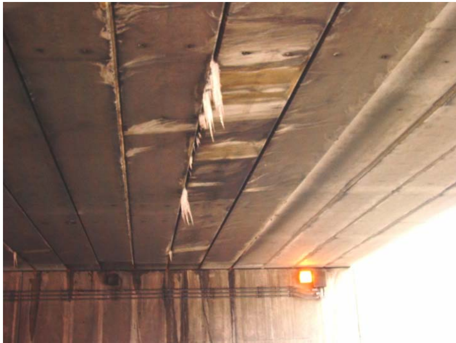
Figure 1.1-2 Deterioration due to lack of adequate post-tensioning in transverse direction.
