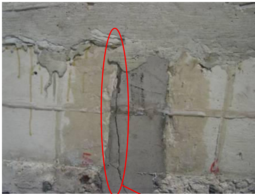
Partial debonding of shear-key
