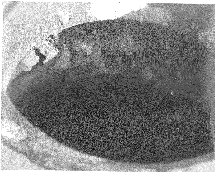
Figure 6. Brick failure. Manhole at Outer Drive and Rotunda Drive. Age 17 years. Brick cracked and displaced. May be due to either frost action or workmanship or both. Brick marked W & F.
