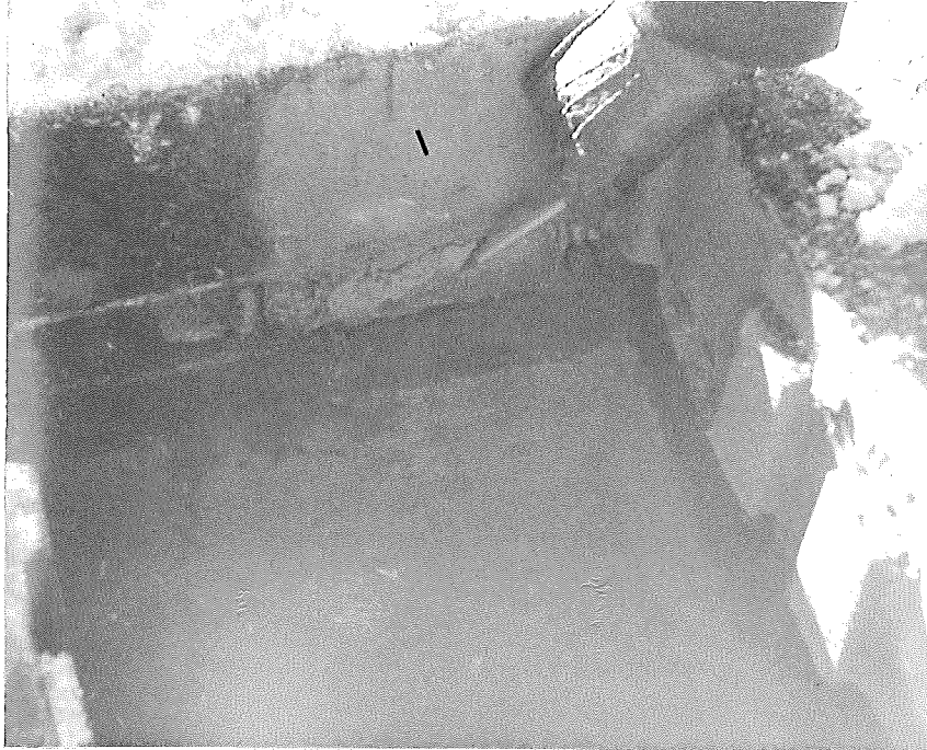
Figure 3. Brick failure by spalling. In catch basin at Pelham Drive and Wabash R.R. grade separation. Daniels Brick. Only one brick in poor condition. Age 7 years.
