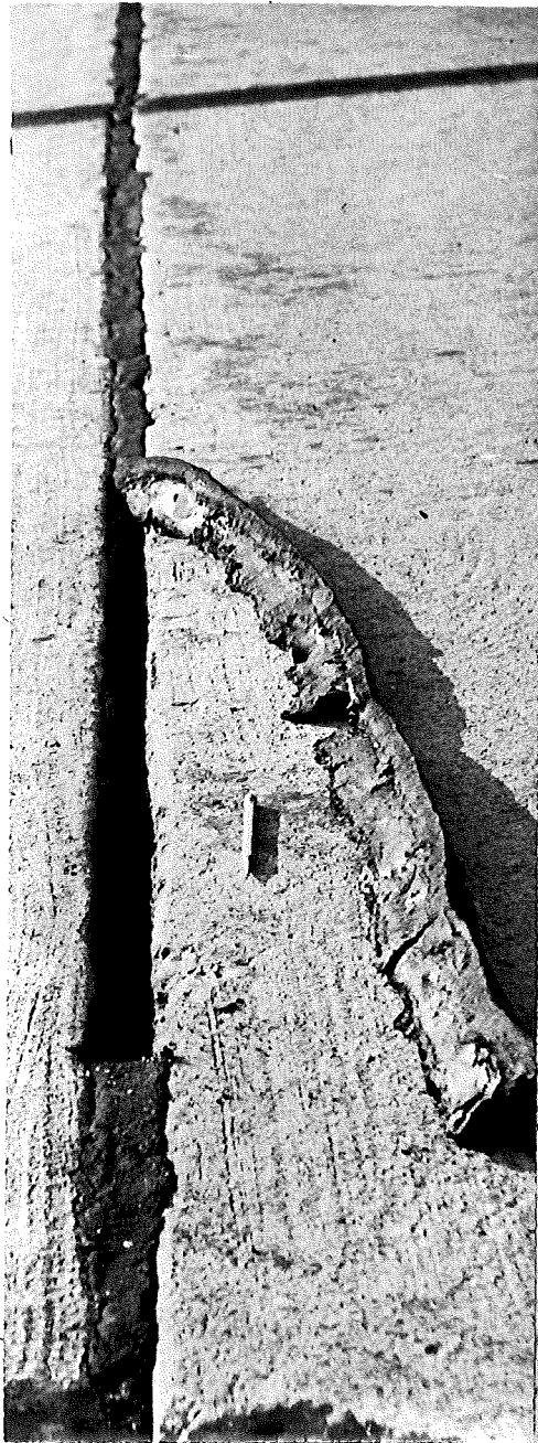
▲ FIGURE 1. TYPICAL JOINT SEAL FAILURE WITH COMPLETE LACK OF ADHESION TO BOTH JOINT FACES. PAVEMENT 7 YRS. OLD. CONSTR. PROJ. F 17-7, C 6. STA. 1171 + 00.
