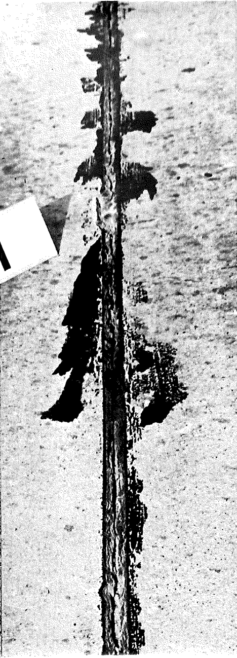
▲ FIGURE 5. LONGITUDINAL FOLD IN JOINT SEAL CONTAINING INFILTRATED FOREIGN MATERIAL. SEALER STILL IN CONTACT BELOW FOLD. CONSTR. PROJ. F19-41, C6. STA. 435+25.
