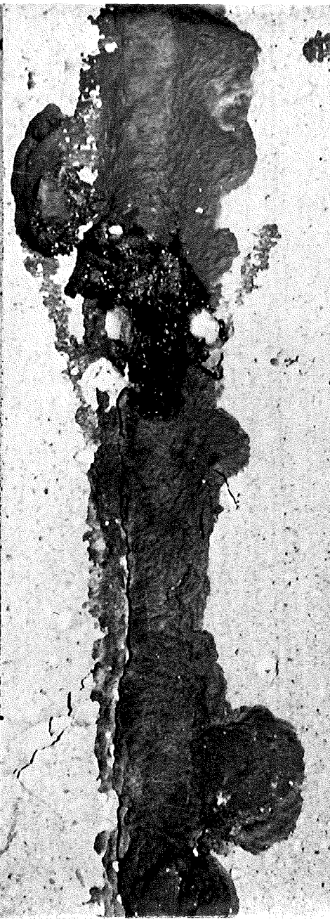
▲ FIGURE 2. PARTIAL ADHESION FAILURE OF JOINT SEAL. NOTE LACK OF ADHESION TO LEFT FACE OF JOINT. PAVEMENT SEALED ONE WEEK. CONSTR. PROJ. 39-45, C 2 AND 3.
