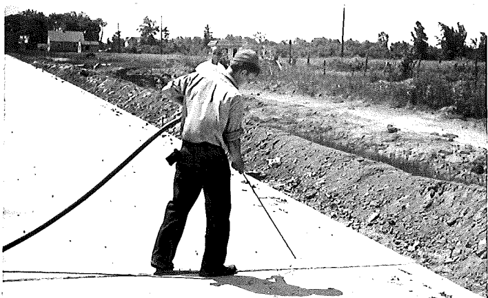
FIGURE 14. BLOWING OUT JOINT WITH COMPRESSED AIR PRIOR TO SEALING BY SARGENT CONSTRUCTION COMPANY.
