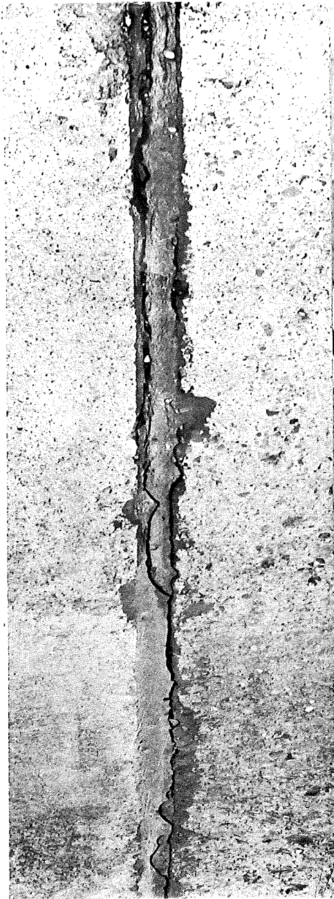
▲ FIGURE 4. FAILURE IN BOTH ADHESION AND COHESION OF JOINT SEAL, US-12.
