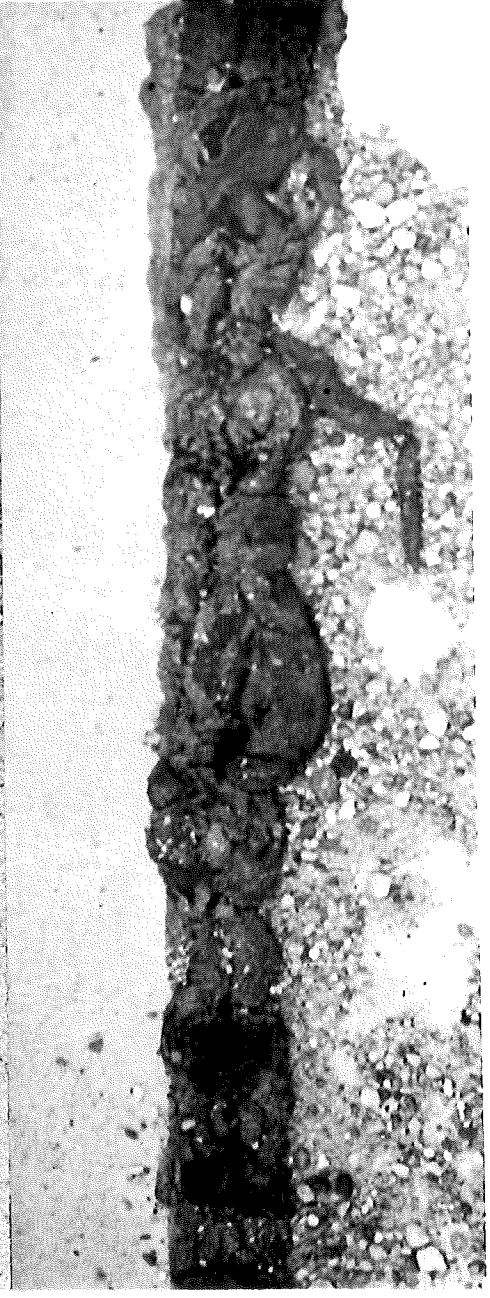
▲ FIGURE 6. NEW CONSTRUCTION NOT YET OPENED TO TRAFFIC IN WHICH SEALER HAS BECOME TOUGH AND FISSURED. CONSTR. PROJ. 39-40, C 4. STA. 981+60.
