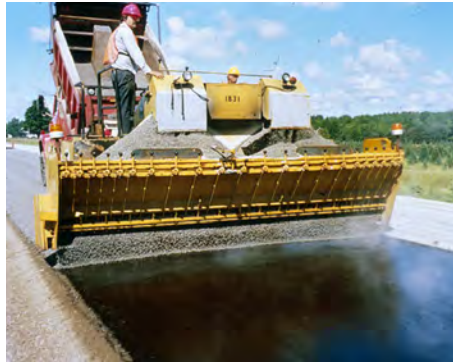
A chip seal improves skid resistance and seals fine surface cracks to reduce water infiltration.
