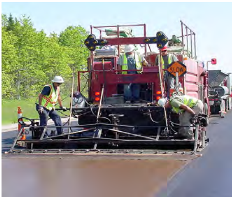
Microsurfacing is the application of a mixture of asphalt emulsion, aggregate and other additives to improve skid resistance.
