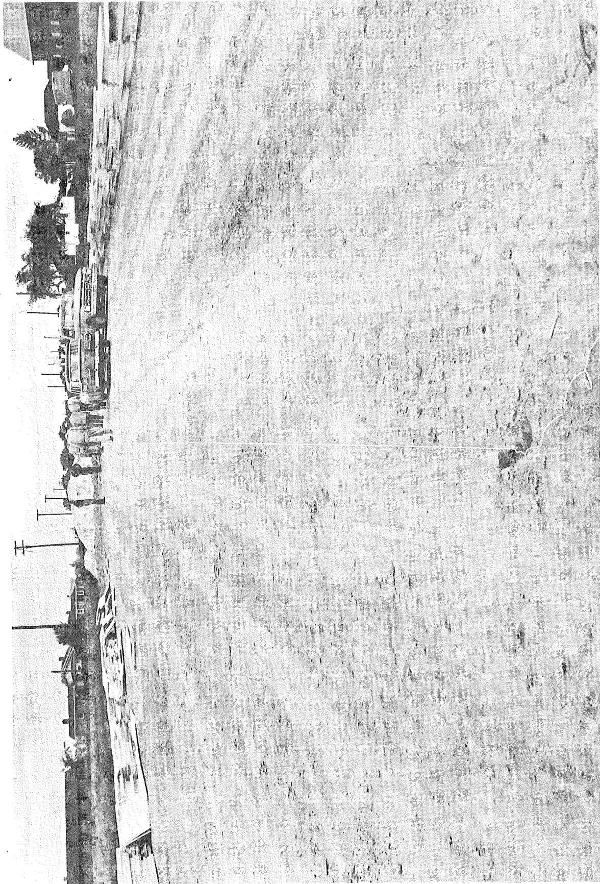
Figure 2. Appearance of prepared subgrade immediately before Styrofoam placement; note stringline used for alignment of Styrofoam sheets.
