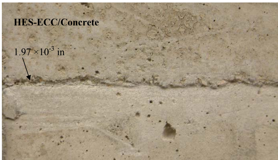
Figure 5.12: Interface delamination of layered repair systems
