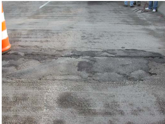
Figure 9.2: Bridge deck cracking
