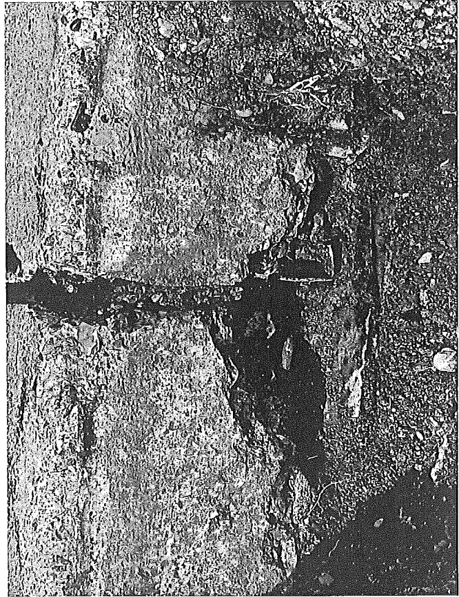
Figure 11. Concrete under neoprene sealed joint at left is sound as contrasted with deteriorated concrete under hot-pour seal at right. Both were installed in 1962 on I 96, Lansing.
