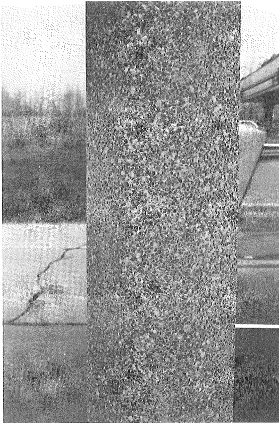
Figure 3. Typical ground polished or etched finish on light pole.
