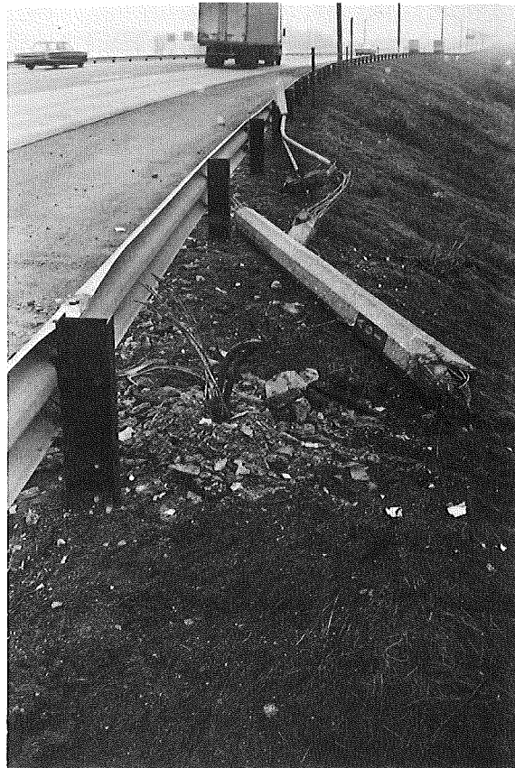
Figure 2. Fallen light pole I 96 near Intersection with US 131. Note dent in top of guardrail where pole fell onto pavement.
